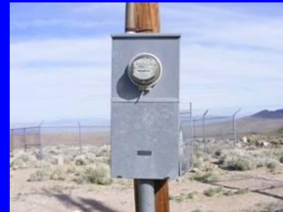
Service-Disconnect Panel Mounted on Utility Pole
