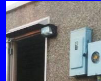
Exterior Light Near Access Door
