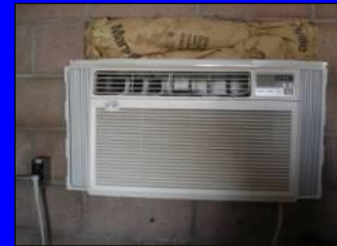
Consumer Grade Air Conditioner Units are not Permitted
