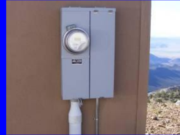
Shelter-mounted Meter and Service-Disconnect Panel
