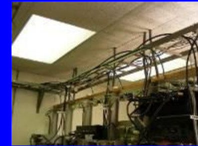
Lights In Front and Behind Equipment Racks
