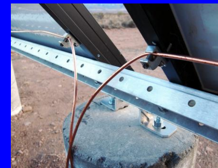
Solar Panels Bonded with #6 AWG Minimum
