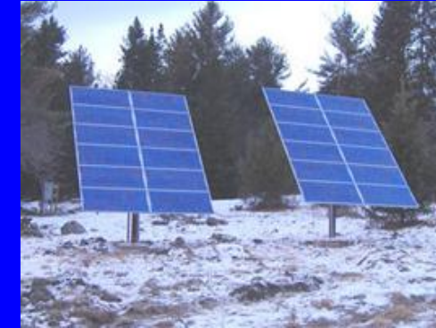
Pole-mounted Solar Panels
