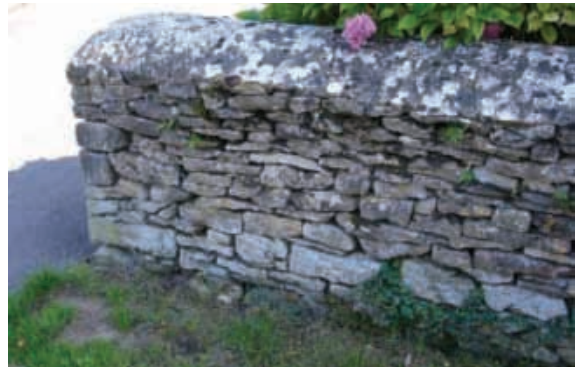
Heaped mortar forms coping
