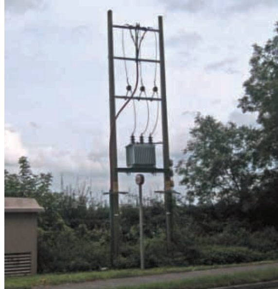
Transformer adjacent to Fir Tree Farm.
