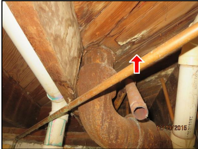
6.3 Item 2(Picture) Water stains
