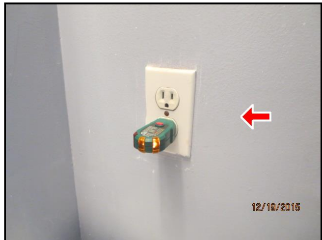
3.3 Item 5(Picture) Non GFCI outlet
