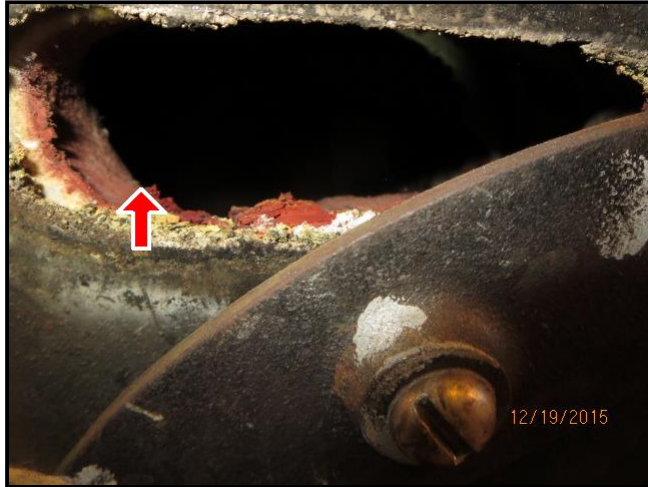
4.0 Item 1(Picture) Firewall cracks
