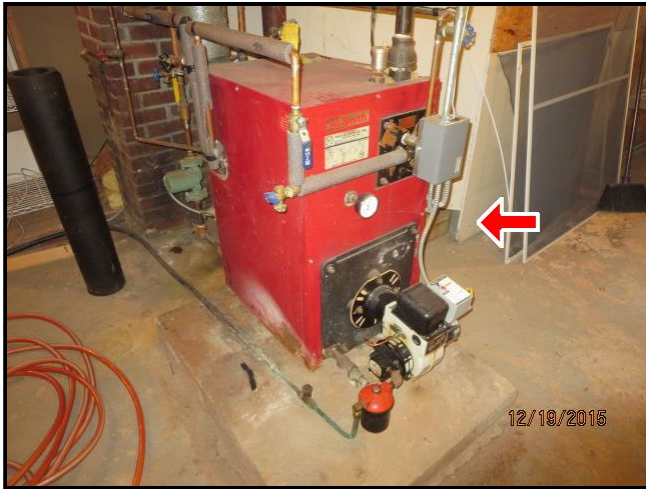
4.0 Item 2(Picture) Boiler
