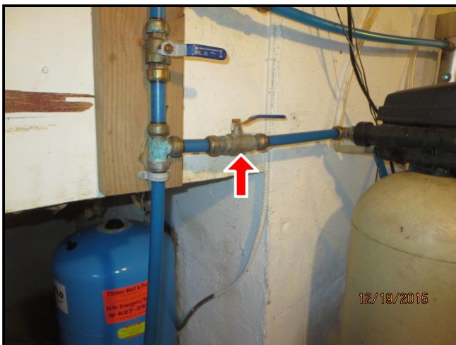
5.3 Item 1(Picture) Main water shut off
