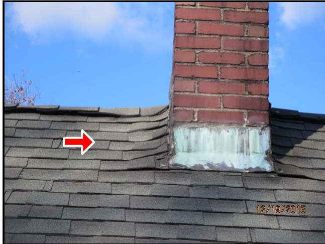
1.0 Item 5(Picture) Tile Lifts
