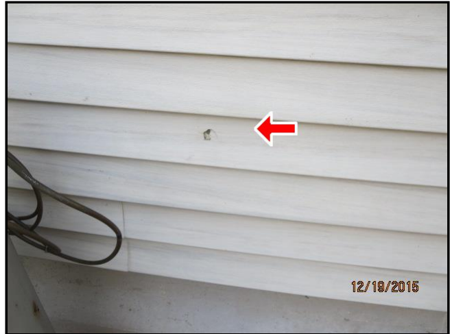
2.0 Item 2(Picture) Damaged Siding
