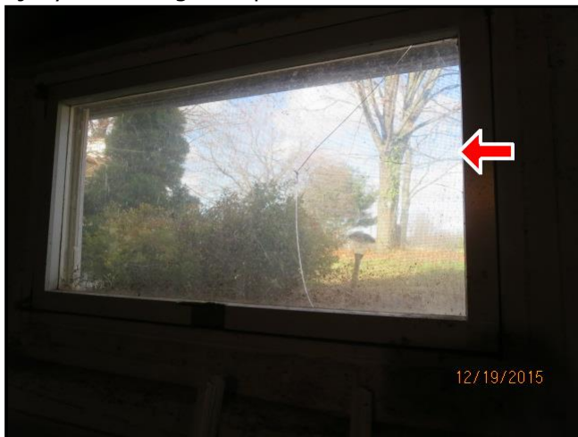
7.6 Item 1(Picture) Cracked glass
