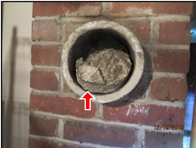
4.5 Item 2(Picture) Possible asbestos
