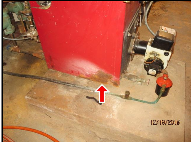
4.0 Item 3(Picture) Boiler Rust
