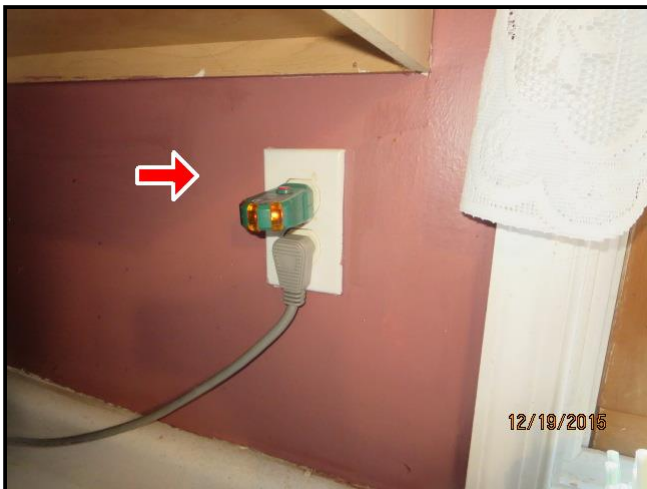
3.3 Item 4(Picture) Non GFCI
