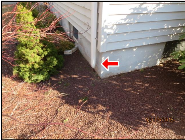
1.2 Item 1(Picture) Needs extension
