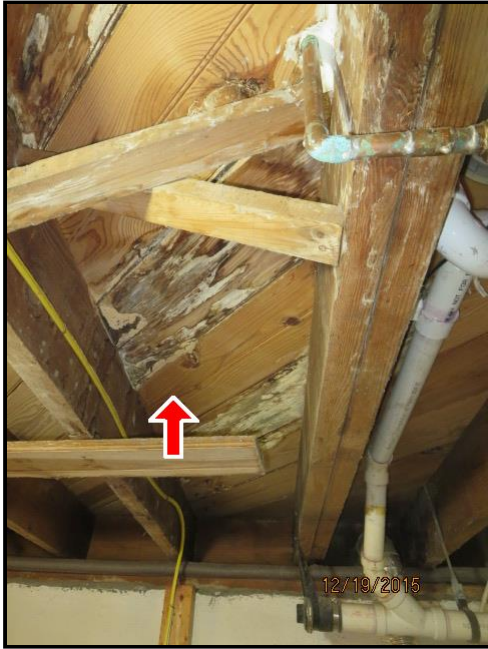
6.3 Item 1(Picture) Water stains
