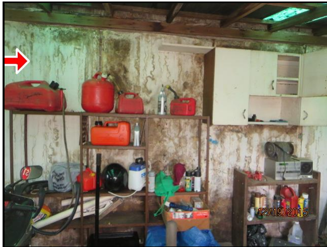
9.0 Item 3(Picture) Water damage & mold
