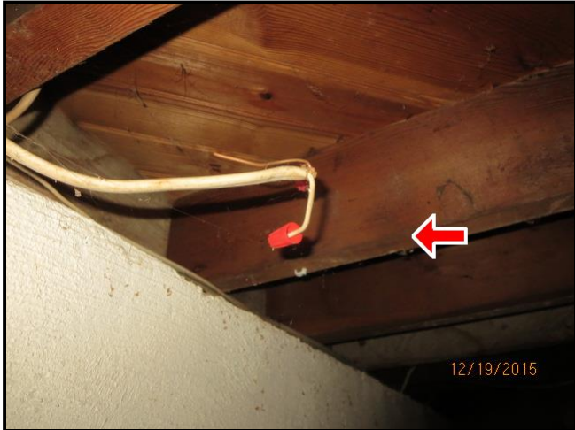
3.3 Item 1(Picture) Exposed wire
