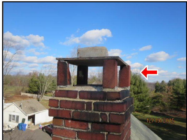
1.1 Item 2(Picture) Needs repair
