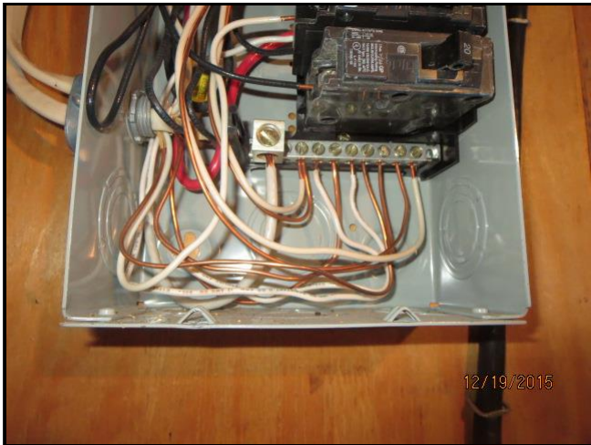
3.1 Item 3(Picture) Sub Panel
