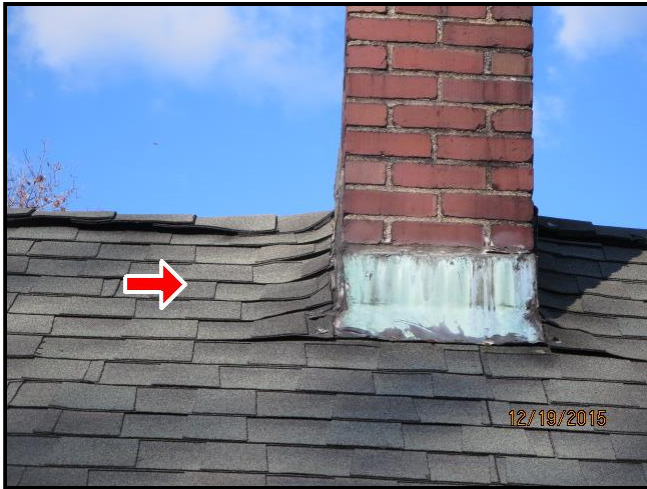
1.0 Item 5(Picture) Tile Lifts
