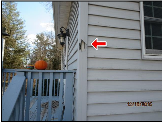
2.0 Item 1(Picture) Damaged Siding
