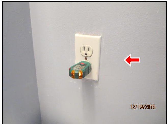
3.3 Item 5(Picture) Non GFCI outlet
