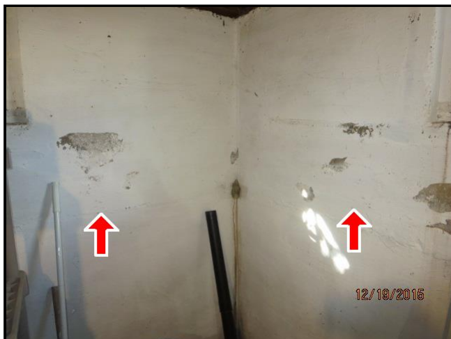
6.0 Item 1(Picture) Efflorescence
