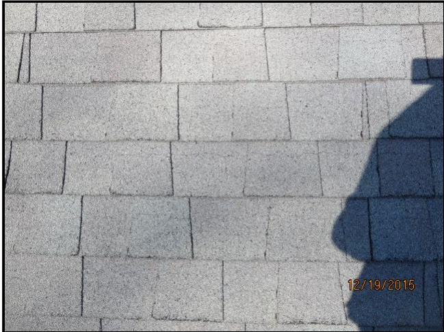
1.0 Item 1(Picture) Cracks
