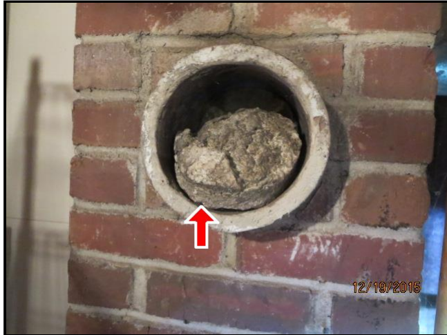
4.5 Item 2(Picture) Possible asbestos
