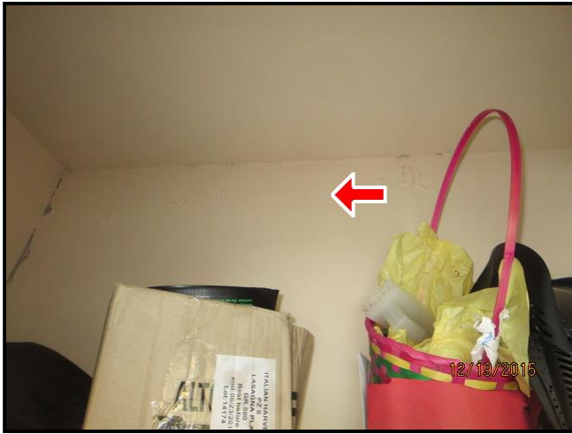
7.1 Item 1(Picture) Possible Led paint
