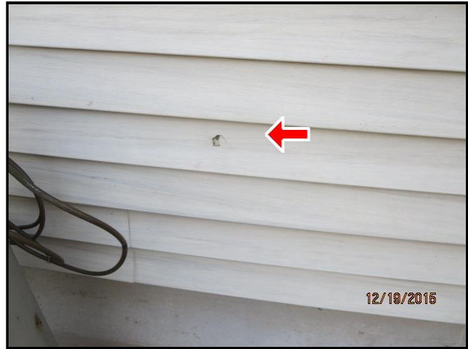
2.0 Item 2(Picture) Damaged Siding
