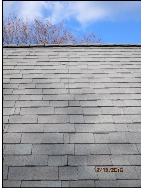
1.0 Item 2(Picture) Buckling
