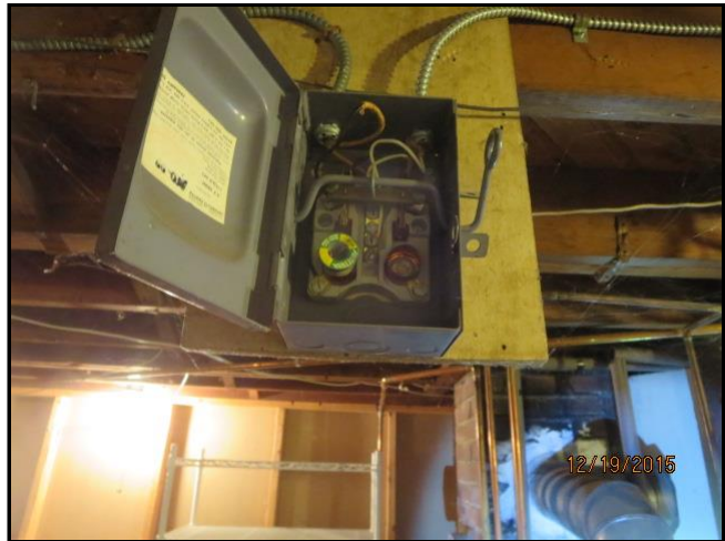
3.1 Item 4(Picture) Open fuse
