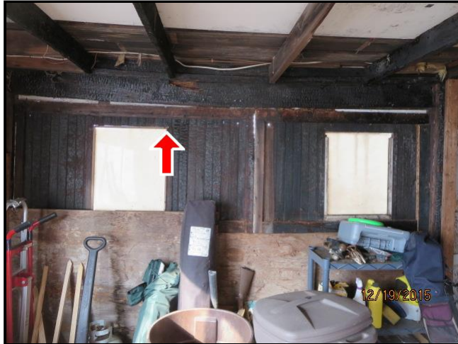
9.0 Item 1(Picture) Burnt beams
