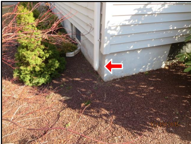
1.2 Item 1(Picture) Needs extention
