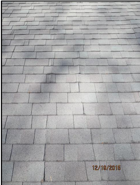
1.0 Item 3(Picture) Buckling Tiles
