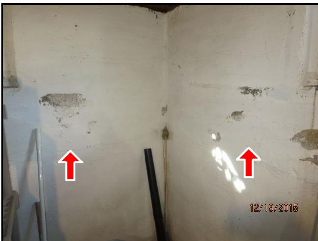
6.0 Item 1(Picture) Efflorescence
