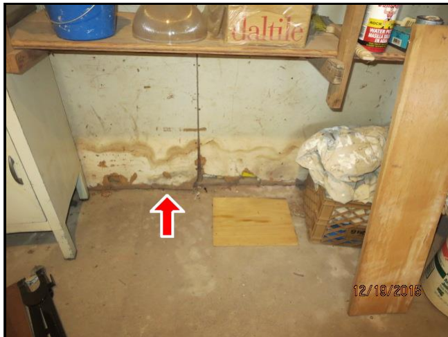
7.1 Item 2(Picture) Water Stain wall
