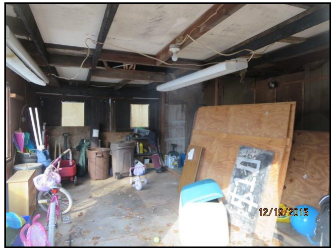
9.0 Item 2(Picture) Burnt areas
