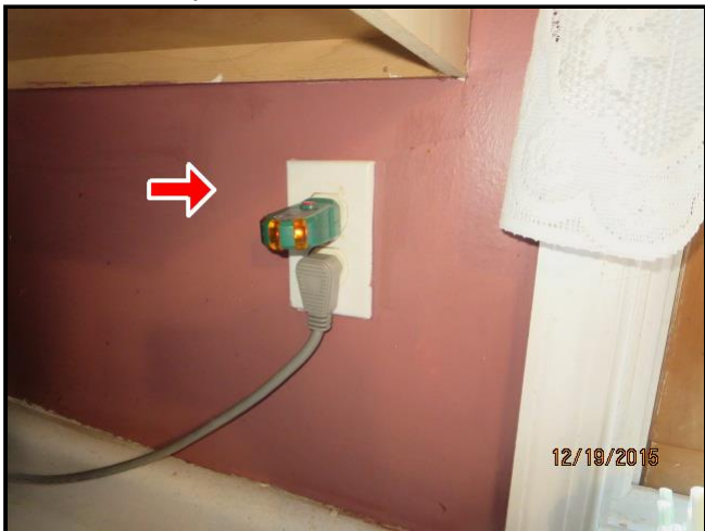
3.3 Item 4(Picture) Non GFCI
