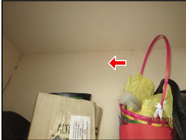
7.1 Item 1(Picture) Possible Led paint
