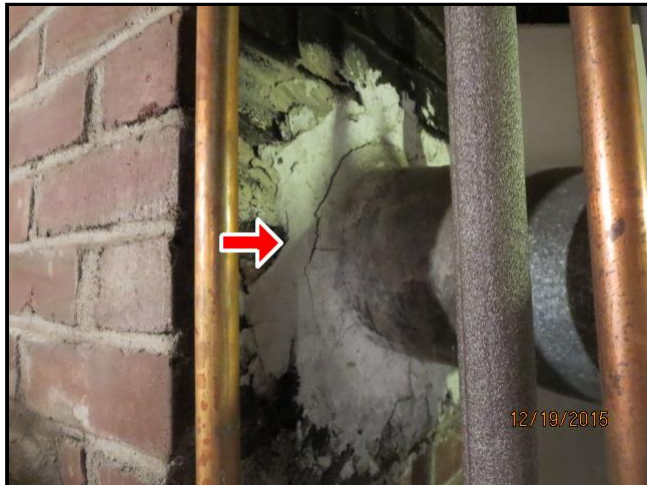
4.5 Item 1(Picture) Needs sealant
