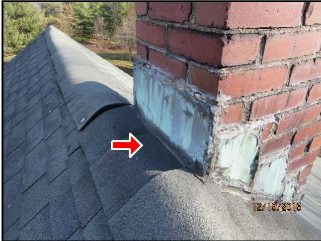
1.1 Item 1(Picture) Flashing
