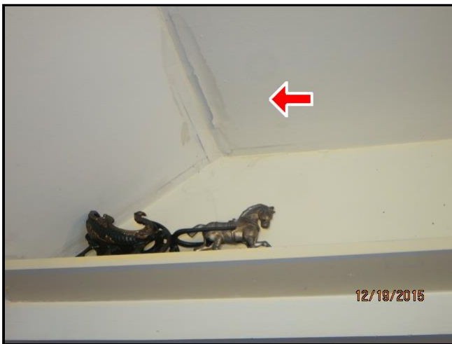
7.0 Item 1(Picture) Water stain
