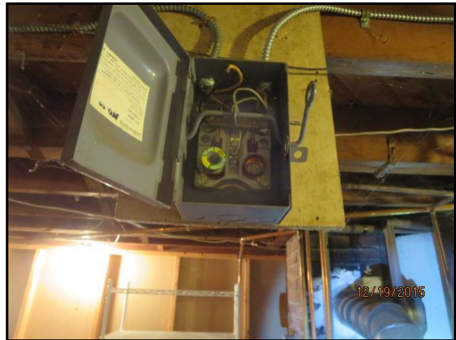
3.1 Item 4(Picture) Open fuse
