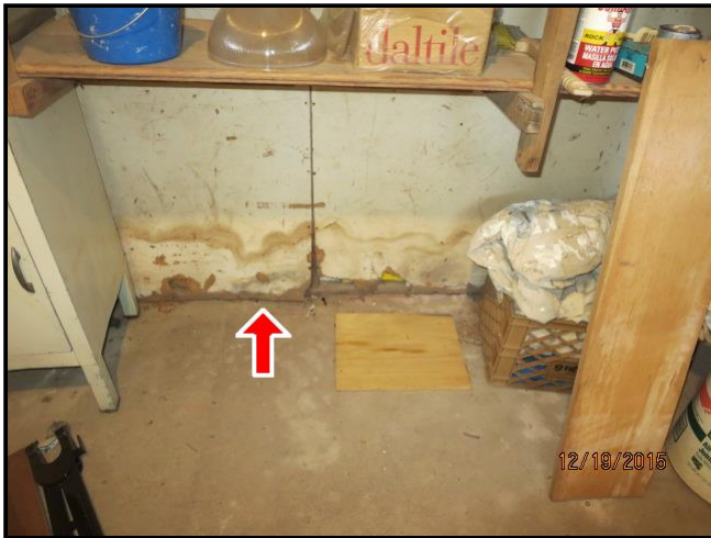
7.1 Item 2(Picture) Water Stain wall
