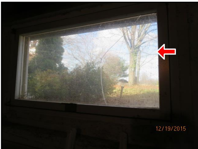
7.6 Item 1(Picture) Cracked glass
