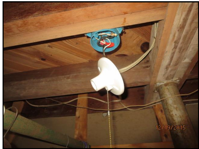
3.3 Item 2(Picture) Exposed wire
