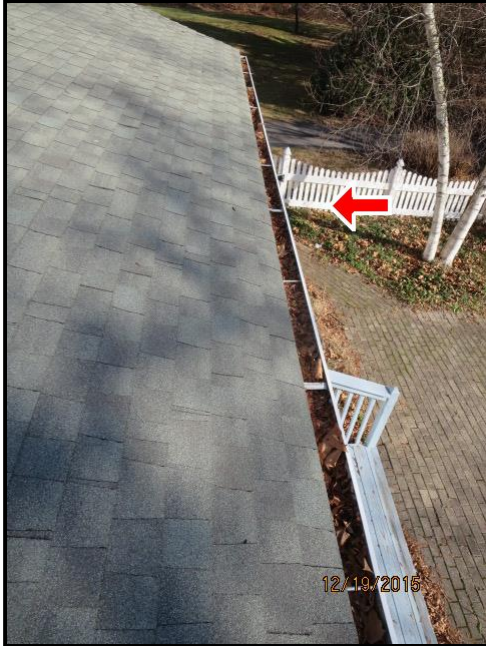
1.2 Item 2(Picture) Clogged Gutters
