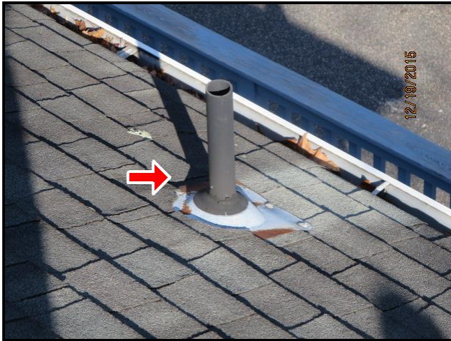
1.3 Item 1(Picture) Failed Boot
