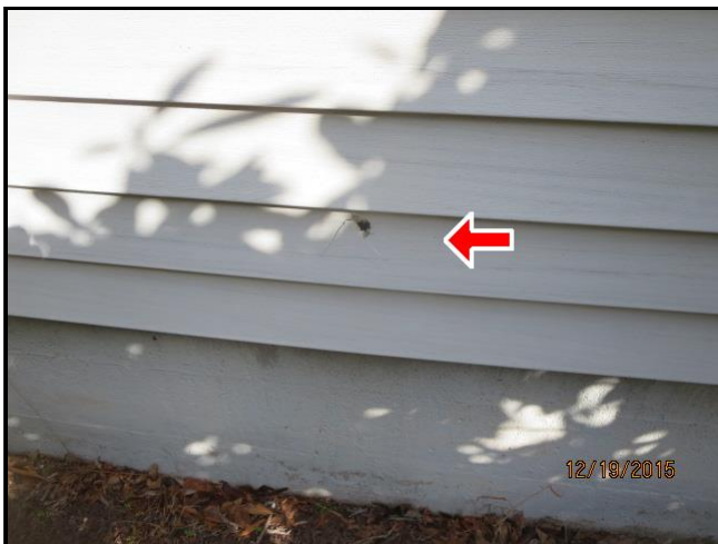
2.0 Item 3(Picture) Damaged siding
