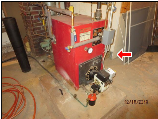
4.0 Item 2(Picture) Boiler
