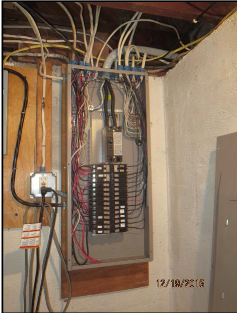
3.6 Item 1(Picture) Main Panel
