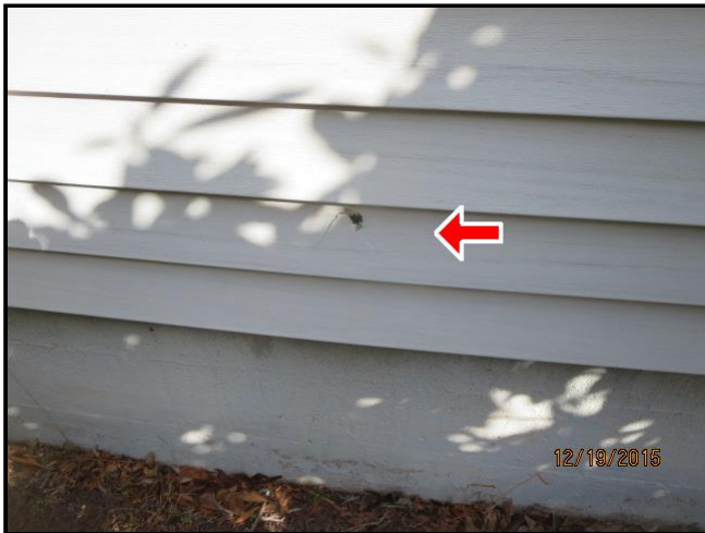
2.0 Item 3(Picture) Damaged siding
