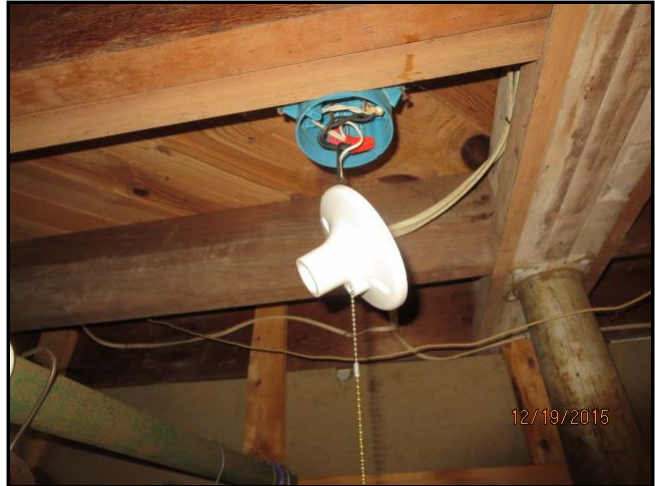
3.3 Item 2(Picture) Exposed wire
