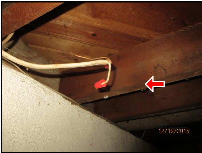
3.3 Item 1(Picture) Exposed wire
