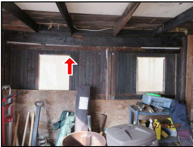
9.0 Item 1(Picture) Burnt beams
