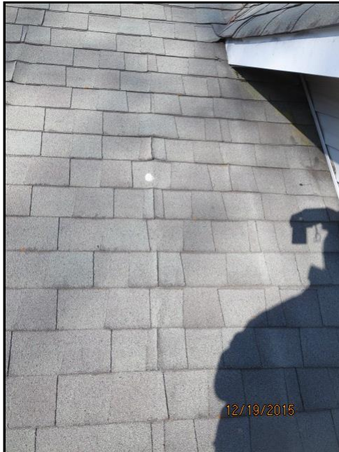
1.0 Item 4(Picture) Buckling Tiles
