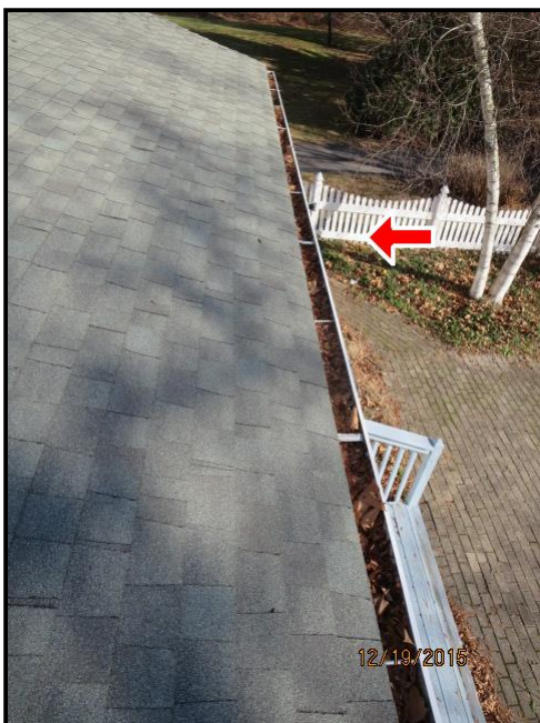
1.2 Item 2(Picture) Clogged Gutters
