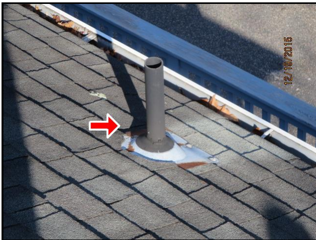
1.3 Item 1(Picture) Failed Boot
