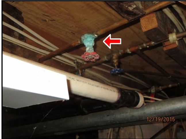
5.1 Item 2(Picture) Corroded valve
