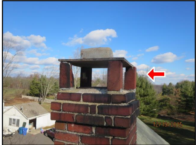
1.1 Item 2(Picture) Needs repair
