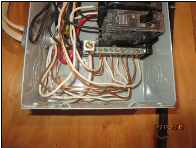
3.1 Item 3(Picture) Sub Panel
