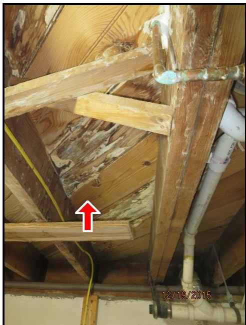
6.3 Item 1(Picture) Water stains
