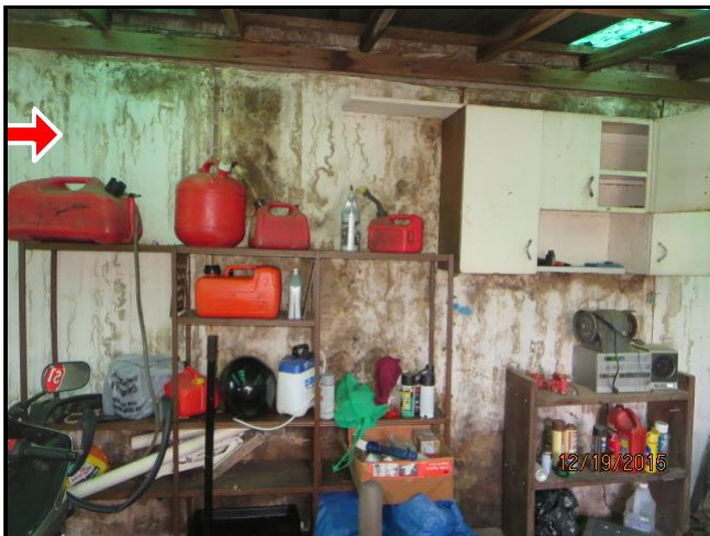
9.0 Item 3(Picture) Water damage & mold
