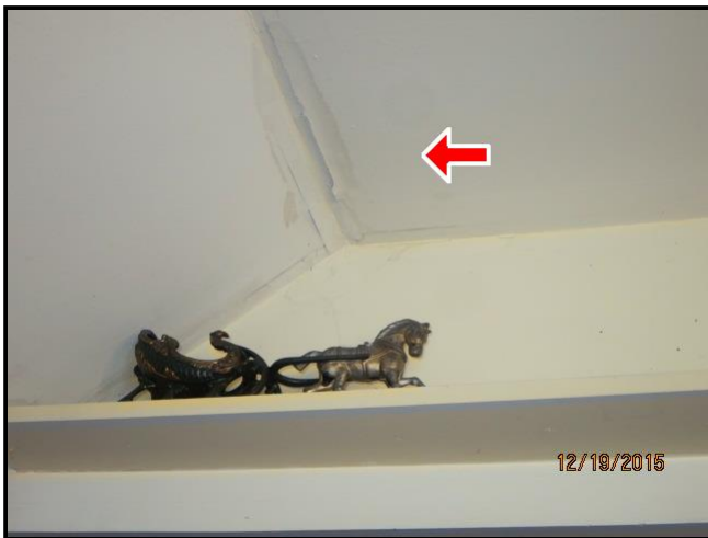
7.0 Item 1(Picture) Water stain
