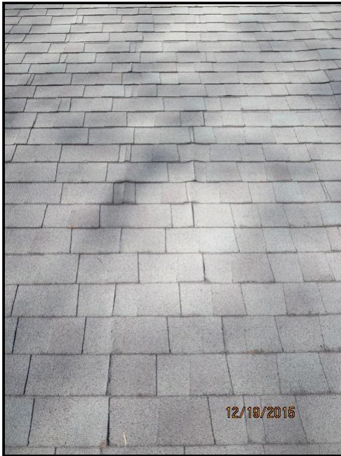
1.0 Item 3(Picture) Buckling Tiles
