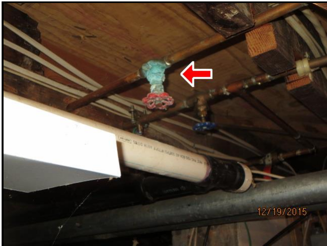
5.1 Item 2(Picture) Corroded valve
