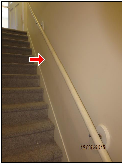
7.3 Item 1(Picture) Loose rail
