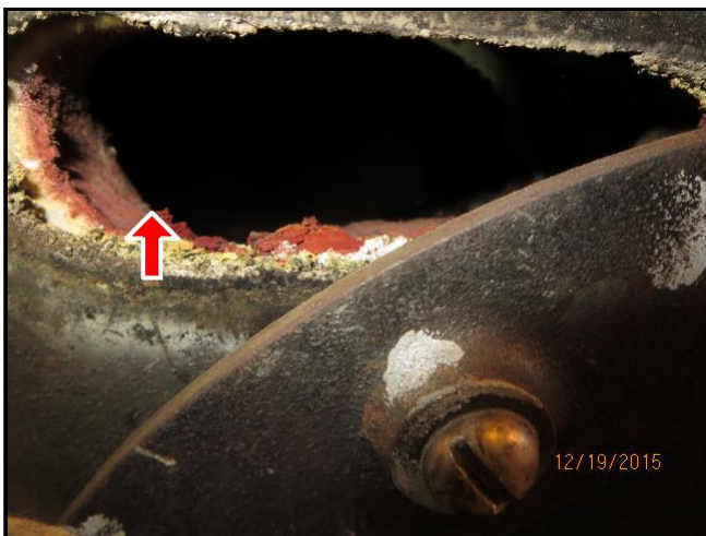
4.0 Item 1(Picture) Firewall cracks
