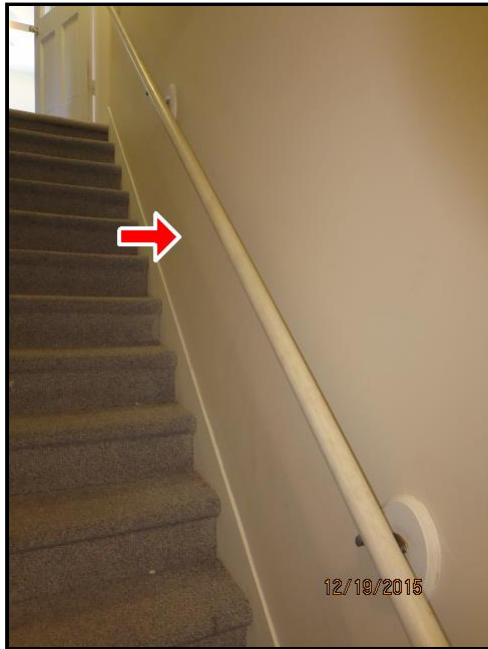
7.3 Item 1(Picture) Loose rail
