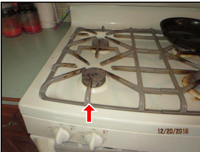
10.1 Item 1(Picture) Not working burner
