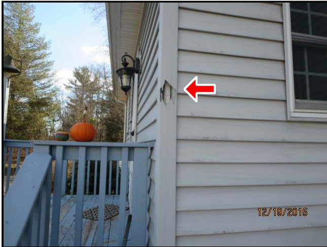
2.0 Item 1(Picture) Damaged Siding
