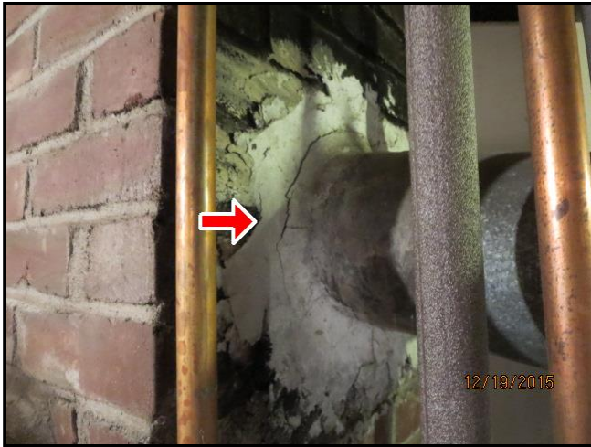
4.5 Item 1(Picture) Needs sealant
