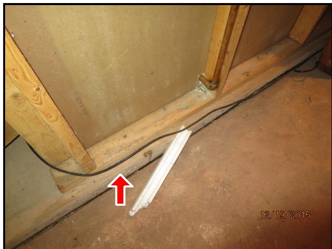
6.1 Item 1(Picture) Base wood
