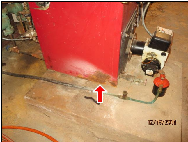
4.0 Item 3(Picture) Boiler Rust
