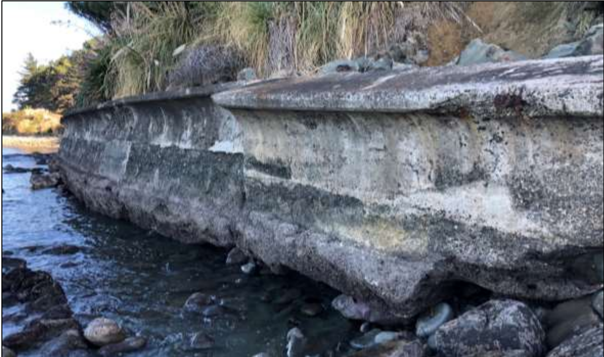
Photo 4.12 Undermining of the remaining seawall
