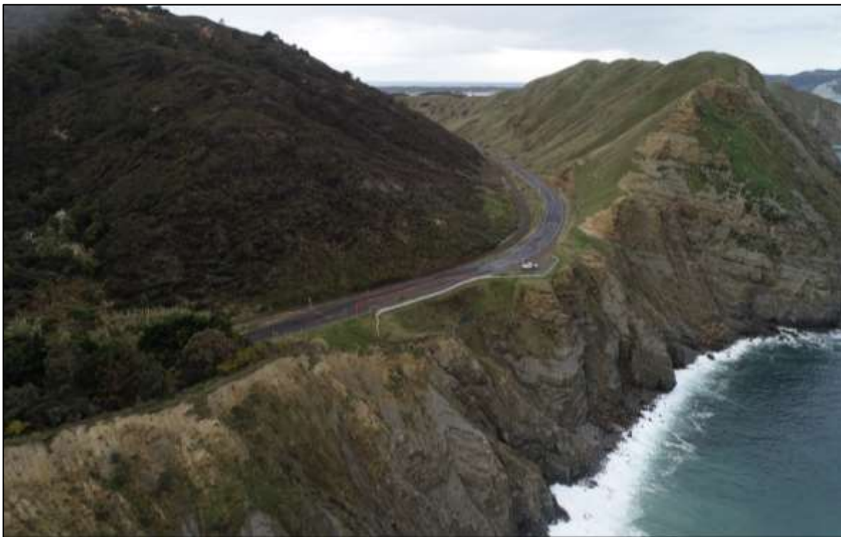
Photo 4.13 Slumping on the Nuhaka-Opoutama Road at 331.4km
