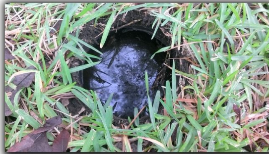
Private shuttle valve box filled with water
