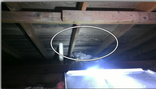
Active water leak in this area
