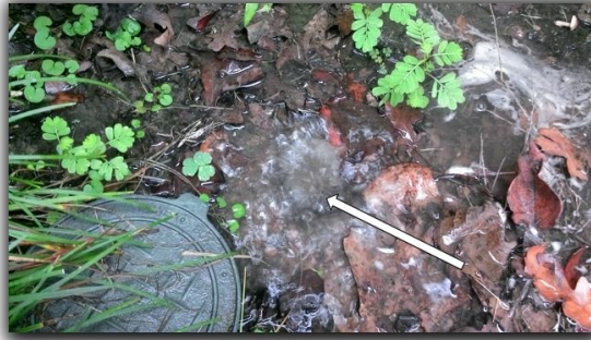
Water leak below hose bib on the south side of the house.
