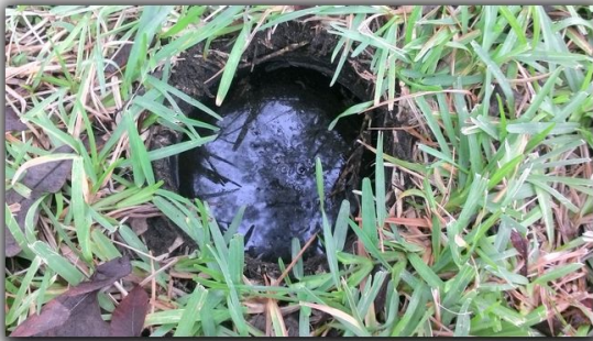
Private shuttle valve box filled with water
