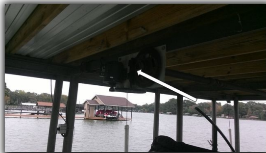
Lift worked intermittently due to under lubrication
