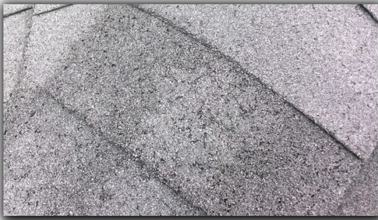
Some granular loss
