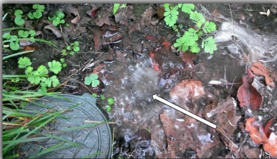
Water leak below hose bib on the south side of the house. The shower diverter in the hall bath is not functioning properly and leaks.
