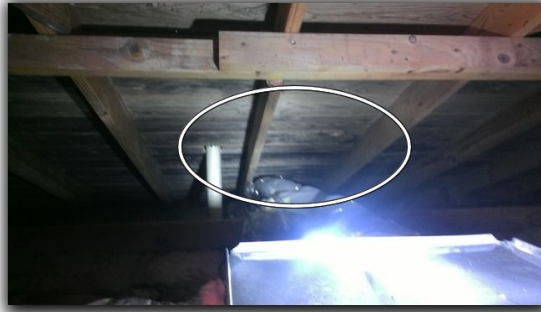
Active water leak in this area
