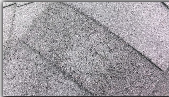
Some granular loss
