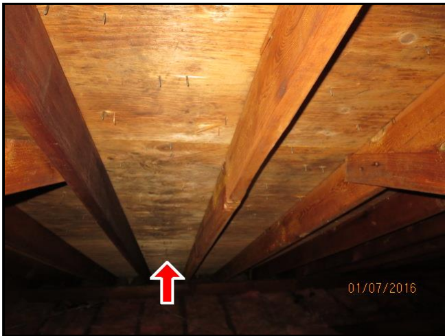
6.5 Item 3(Picture) Possible Mold
