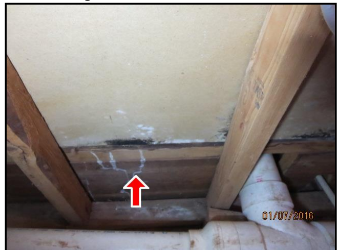
6.0 Item 2(Picture) Possible mold
