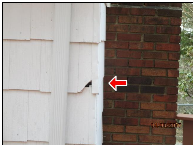
2.0 Item 1(Picture) Damaged siding
