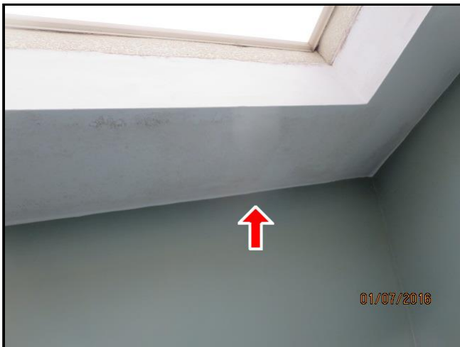
1.2 Item 7(Picture) Possible mold
