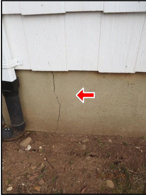
6.1 Item 7(Picture) Foundation crack
