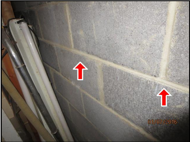
6.1 Item 3(Picture) Crack
