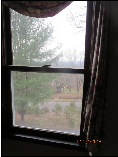
8.6 Item 1(Picture) Non working window
