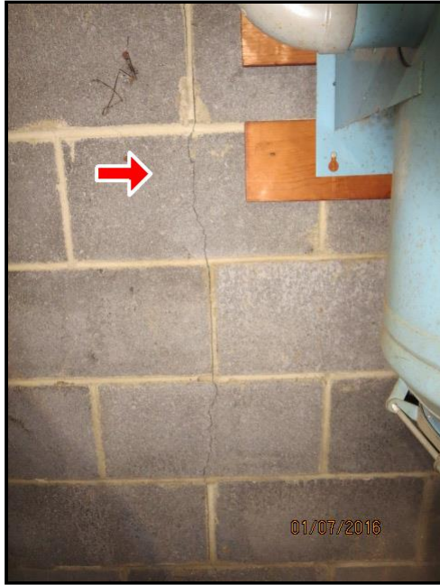
6.1 Item 5(Picture) Crack
