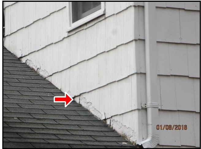
2.0 Item 6(Picture) Damaged siding
