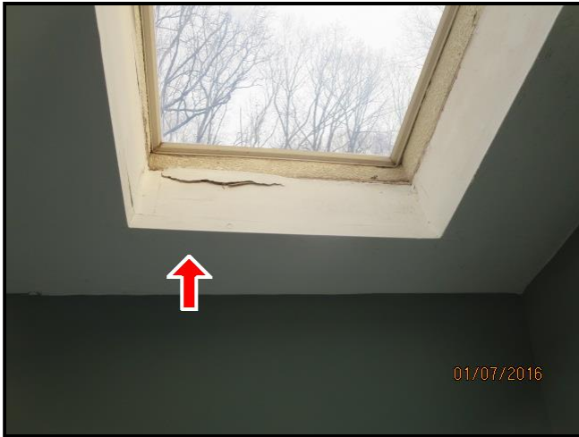
1.2 Item 3(Picture) Skylight damage
