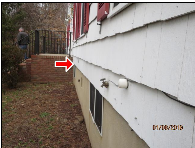
2.0 Item 9(Picture) Buckled siding
