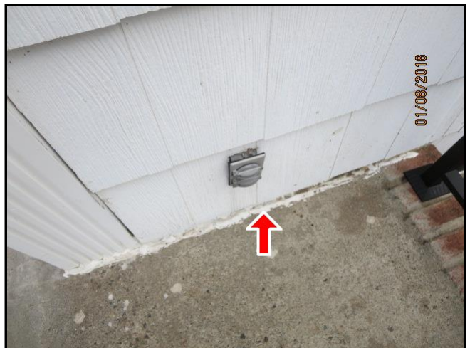
3.3 Item 6(Picture) open ground and loose
