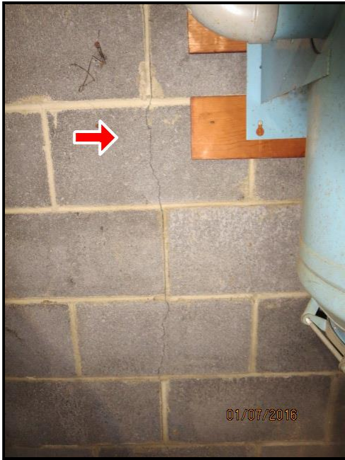
6.1 Item 5(Picture) Crack
