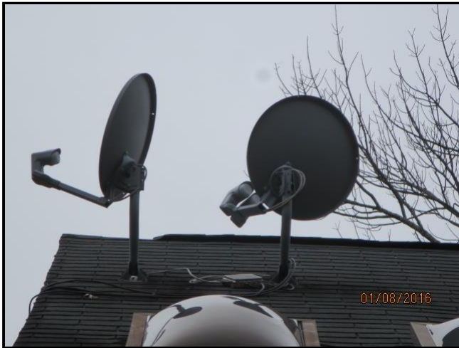
1.2 Item 2(Picture) Satellite dishes
