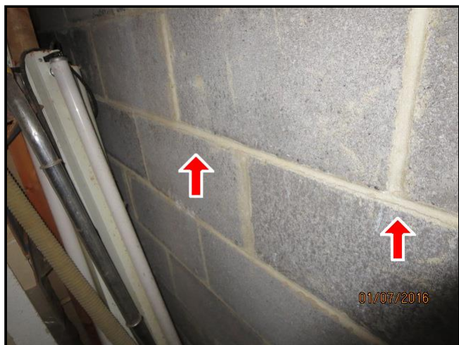
6.1 Item 3(Picture) Crack
