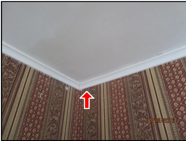
8.0 Item 1(Picture) Water stain
