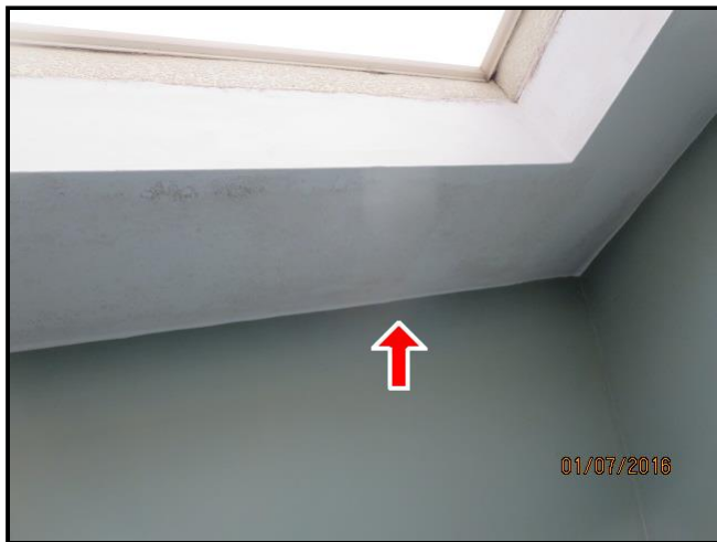
1.2 Item 7(Picture) Possible mold
