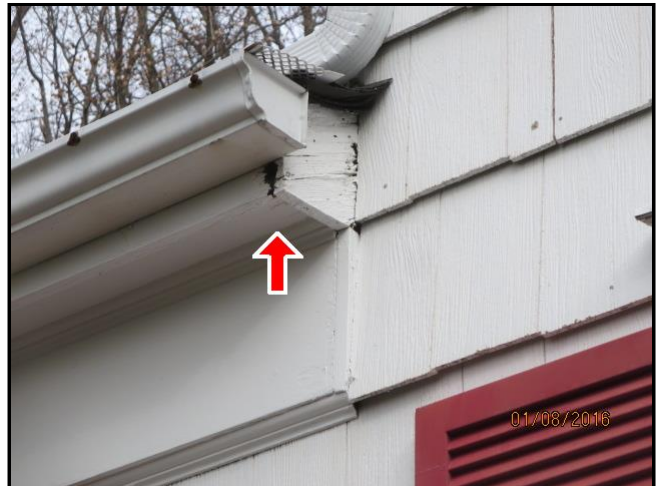
2.0 Item 8(Picture) Rotted trim
