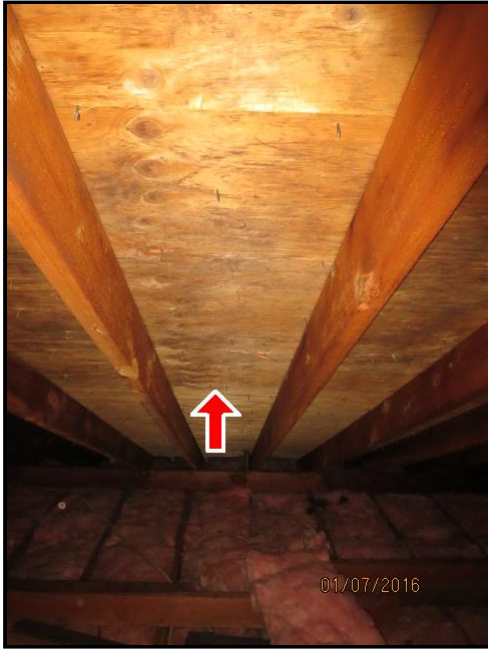
6.5 Item 1(Picture) Possible Mold
