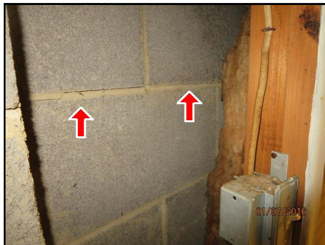
6.1 Item 2(Picture) Crack
