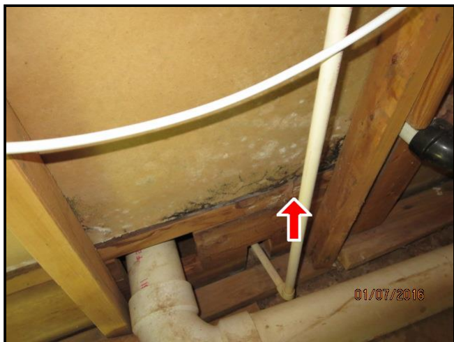
6.0 Item 1(Picture) Possible Mold
