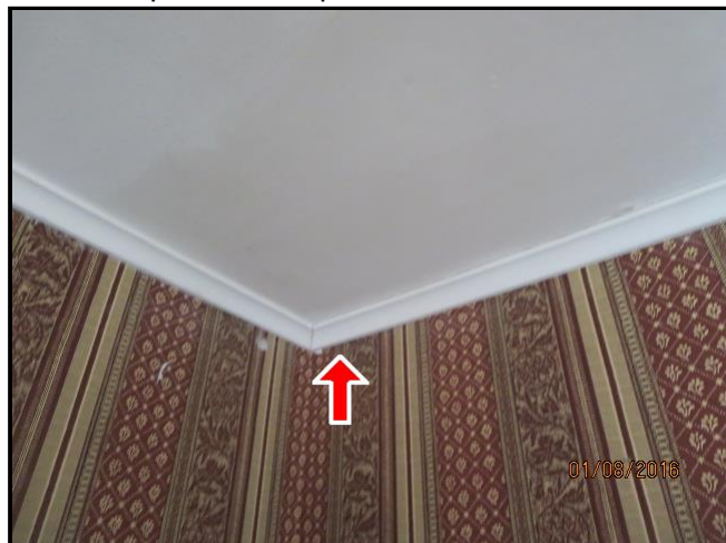
8.0 Item 1(Picture) Water stain
