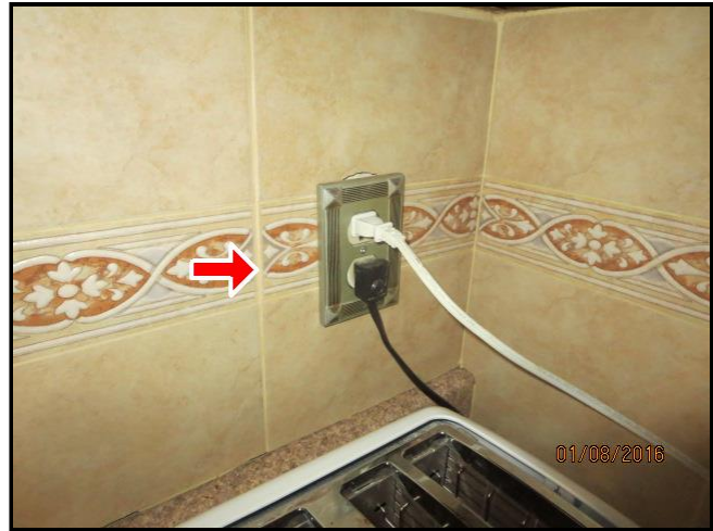
3.3 Item 11(Picture) Non GFCI
