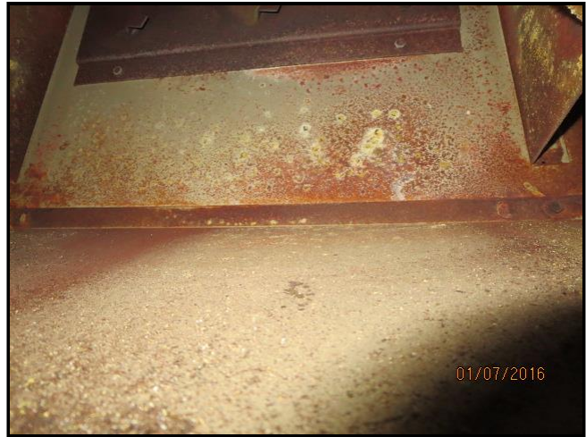
4.0 Item 2(Picture) Rust
