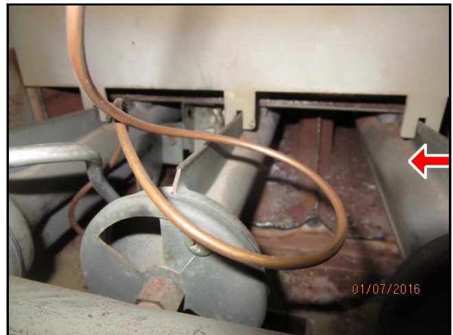
4.0 Item 4(Picture) Rust
