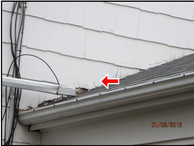
2.0 Item 5(Picture) Damaged siding
