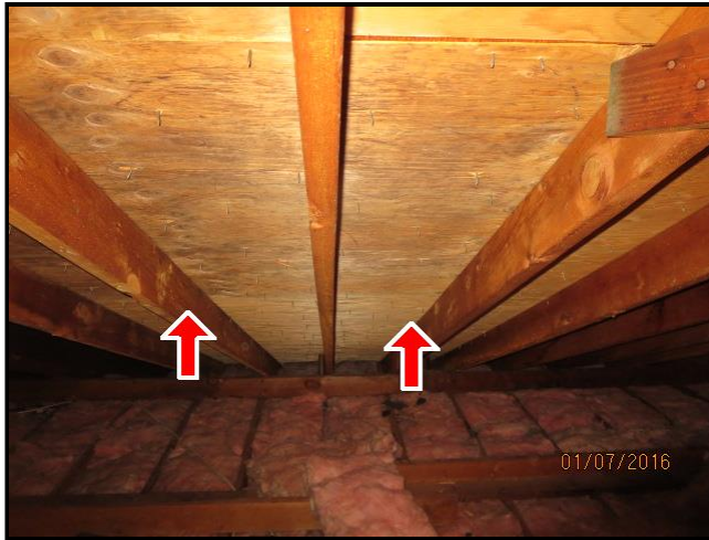
6.5 Item 2(Picture) Possible Mold
