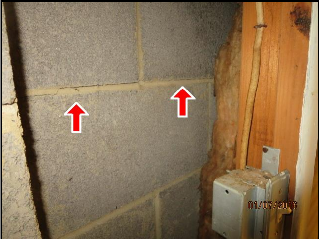
6.1 Item 2(Picture) Crack
