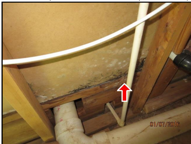
6.0 Item 1(Picture) Possible Mold
