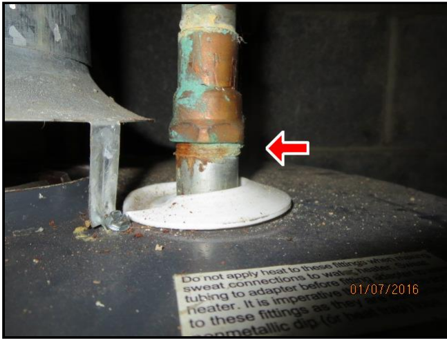
5.1 Item 1(Picture) Pipe corrosion
