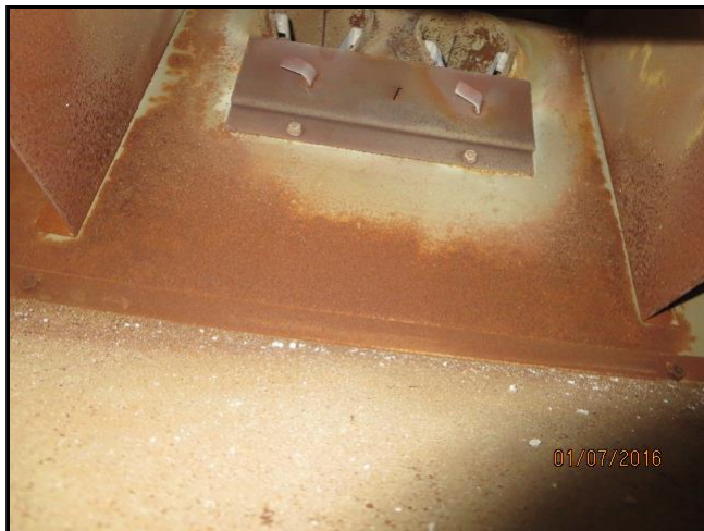
4.0 Item 3(Picture) Rust
