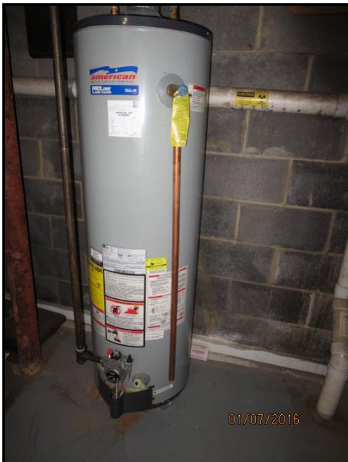
5.2 Item 1(Picture) Water heater
