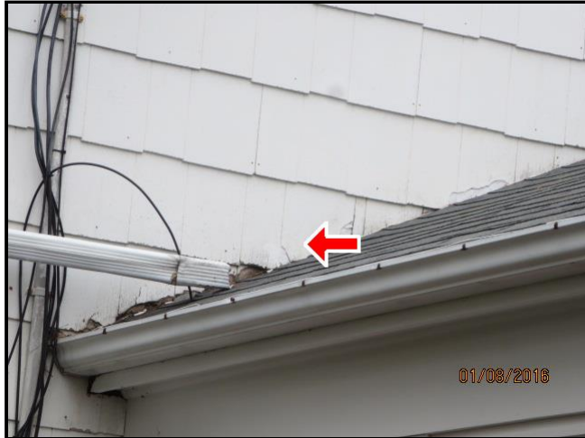
2.0 Item 5(Picture) Damaged siding
