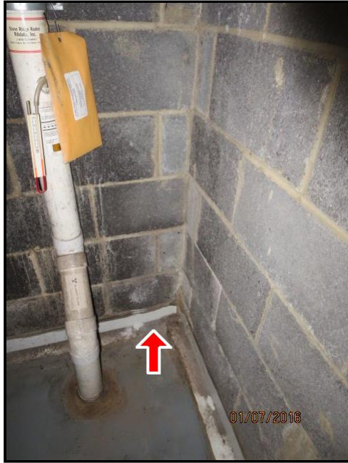
6.0 Item 3(Picture) Efflorescence
