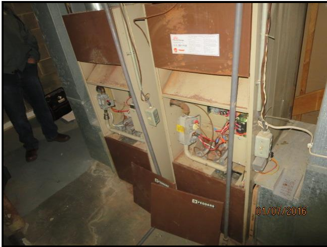
4.0 Item 1(Picture) Rusty Furnaces
