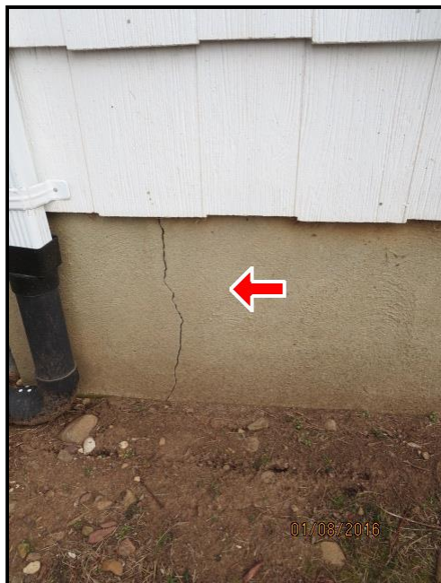
6.1 Item 7(Picture) Foundation crack
