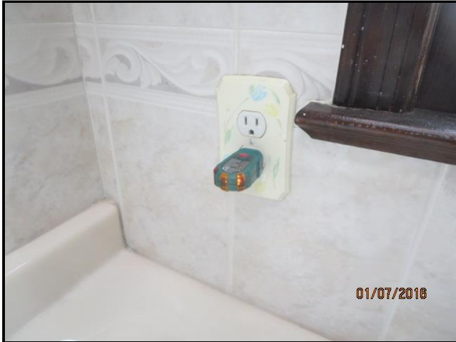
3.3 Item 10(Picture) Non GFCI
