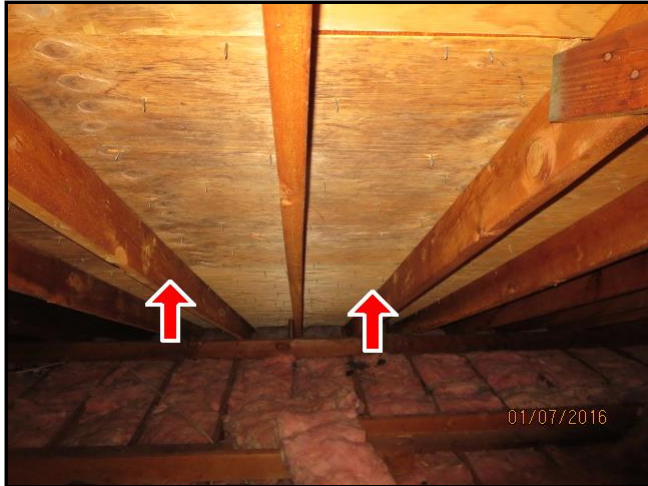
6.5 Item 2(Picture) Possible Mold
