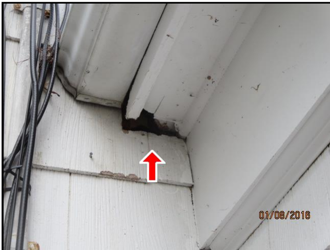
2.0 Item 3(Picture) Hole in siding
