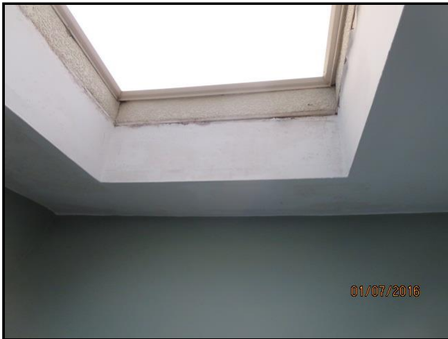
1.2 Item 5(Picture) Damaged skylight
