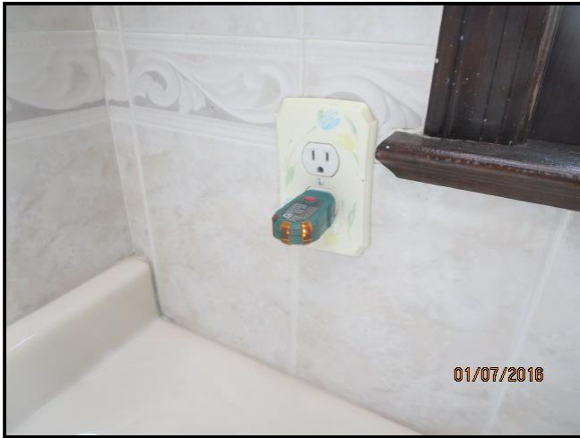
3.3 Item 10(Picture) Non GFCI
