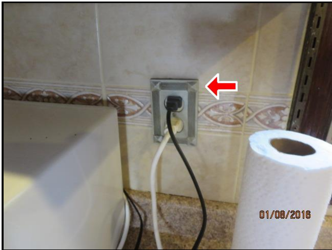
3.3 Item 12(Picture) Non GFCI
