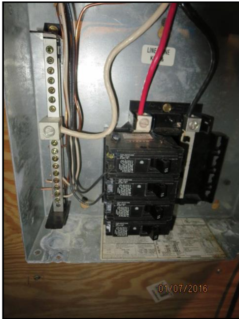
3.1 Item 4(Picture) Sub Panel
