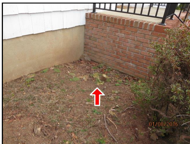
2.4 Item 1(Picture) Negative slope
