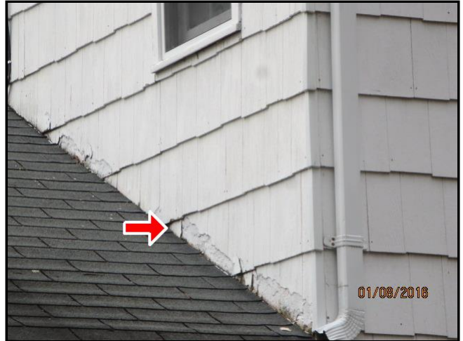
2.0 Item 6(Picture) Damaged siding
