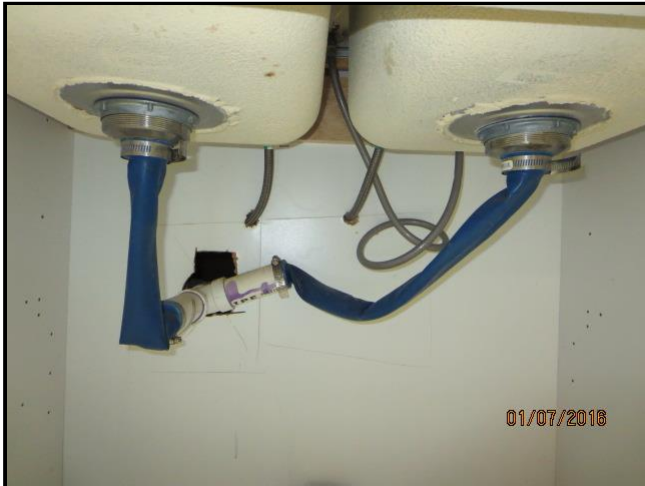
5.0 Item 1(Picture) Missing piping
