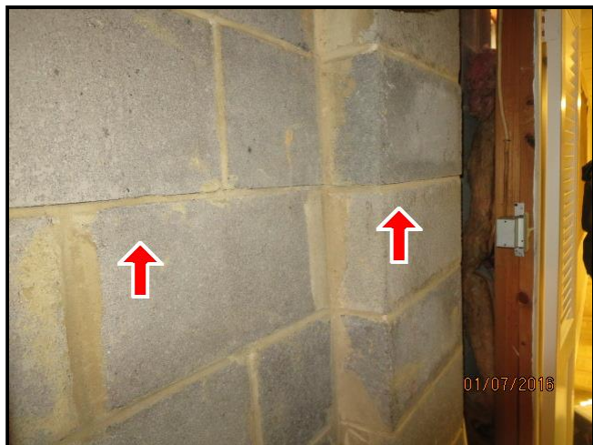
6.1 Item 1(Picture) Crack
