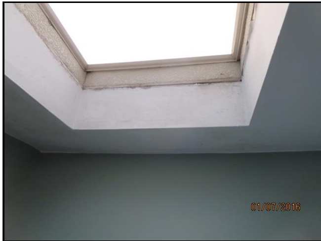
1.2 Item 5(Picture) Damaged skylight
