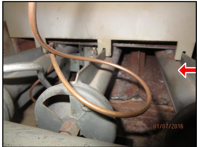
4.0 Item 4(Picture) Rust
