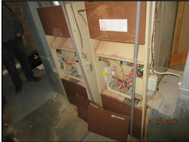
4.0 Item 1(Picture) Rusty Furnaces
