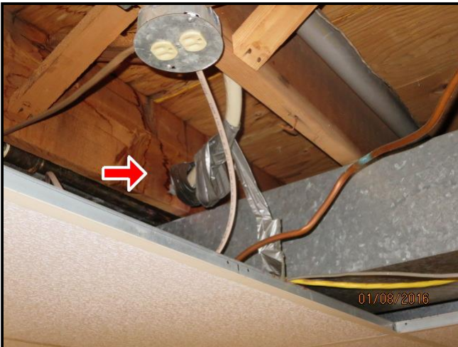
3.3 Item 8(Picture) Open splice
