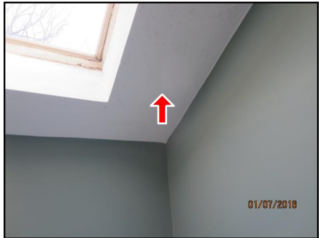
1.2 Item 6(Picture) Possible mold
