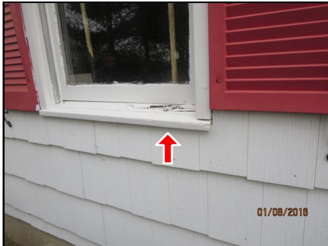
2.0 Item 7(Picture) Rotted trim
