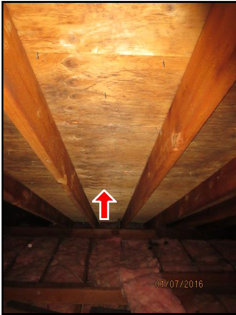
6.5 Item 1(Picture) Possible Mold
