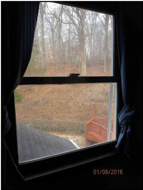
8.6 Item 3(Picture) non working window
