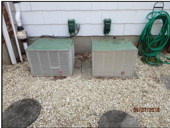
4.8 Item 1(Picture) Condensers
