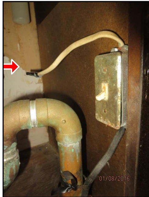
3.3 Item 9(Picture) Open splice
