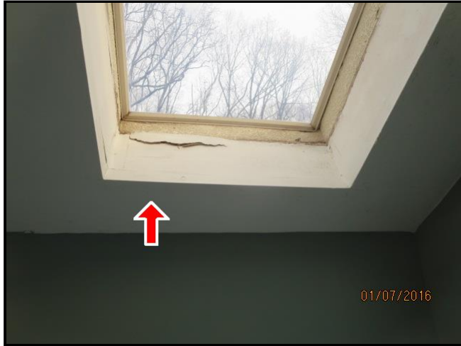
1.2 Item 3(Picture) Skylight damage
