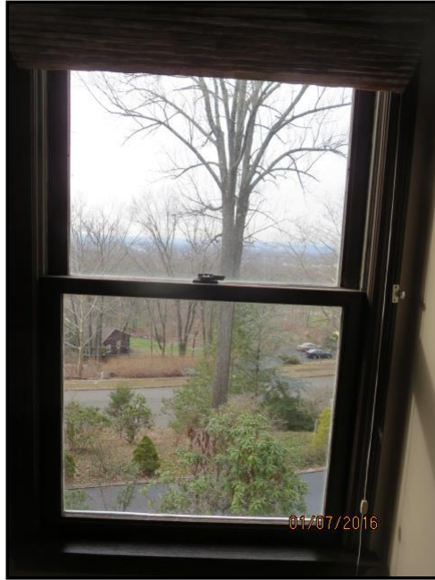
8.6 Item 2(Picture) Non working window
