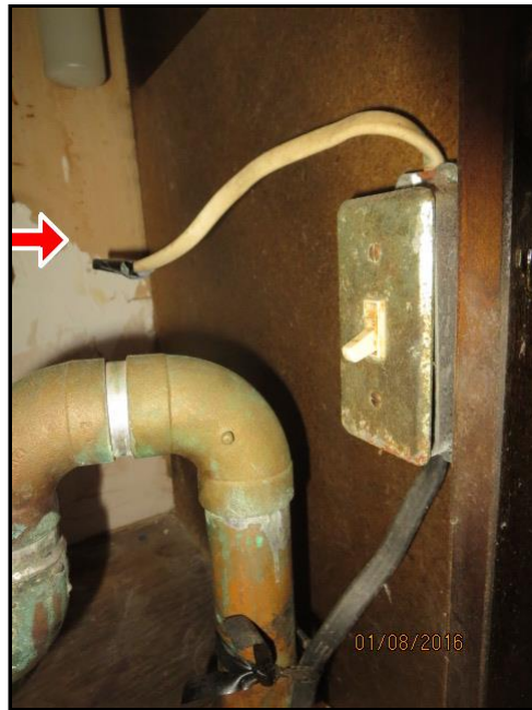
3.3 Item 9(Picture) Open splice
