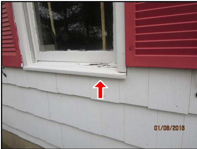
2.0 Item 7(Picture) Rotted trim
