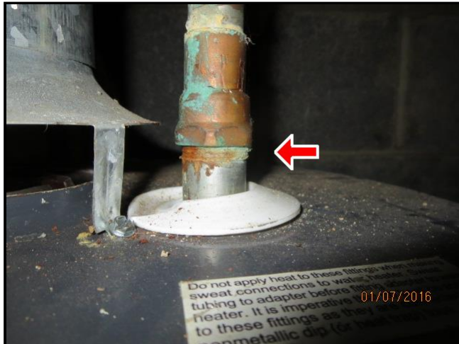
5.1 Item 1(Picture) Pipe corrosion
