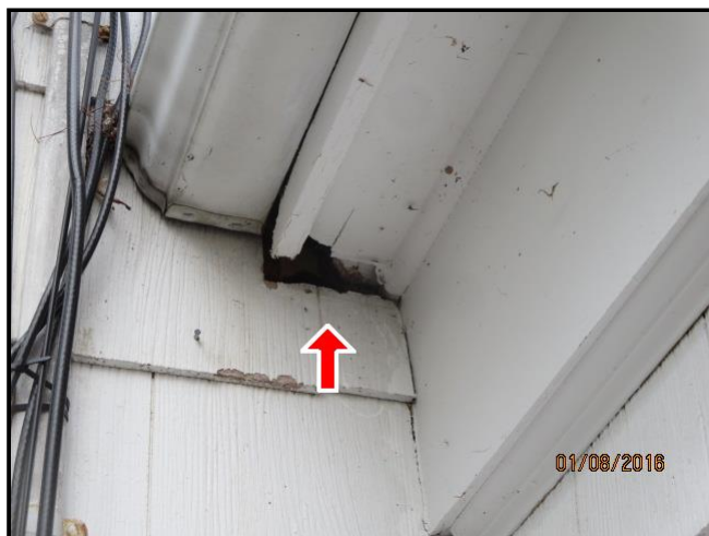
2.0 Item 3(Picture) Hole in siding
