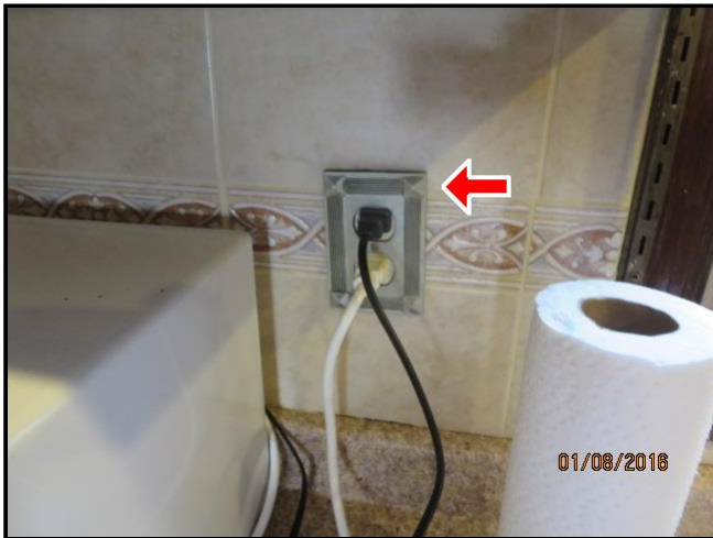
3.3 Item 12(Picture) Non GFCI
