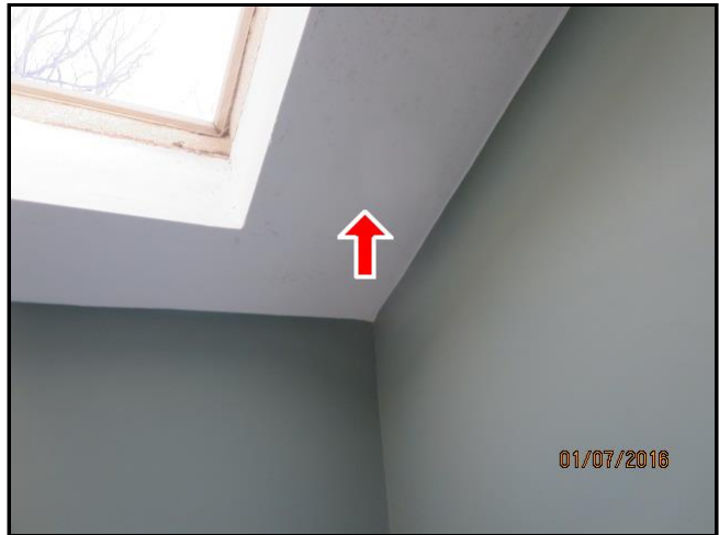
1.2 Item 6(Picture) Possible mold
