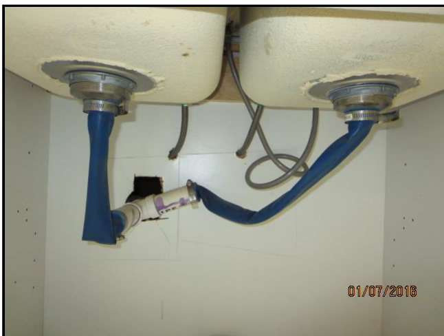
5.0 Item 1(Picture) Missing piping
