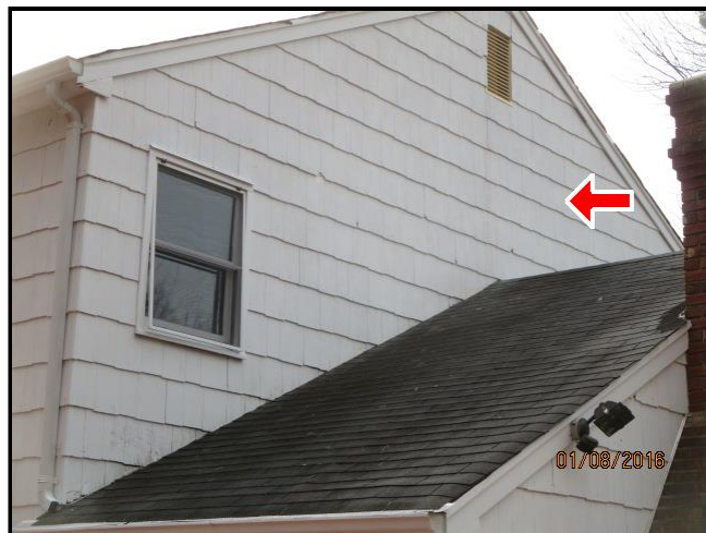
2.0 Item 2(Picture) Damaged siding
