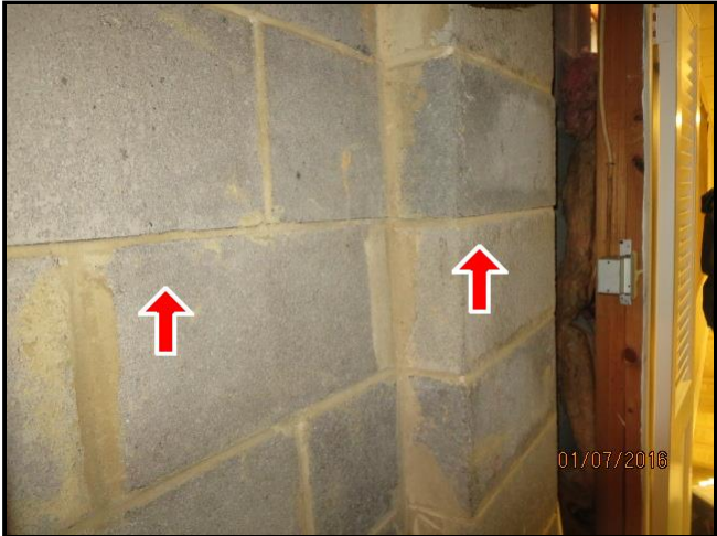
6.1 Item 1(Picture) Crack
