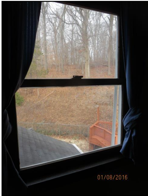
8.6 Item 3(Picture) non working window
