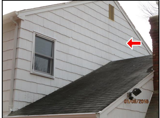
2.0 Item 2(Picture) Damaged siding
