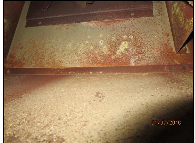
4.0 Item 2(Picture) Rust
