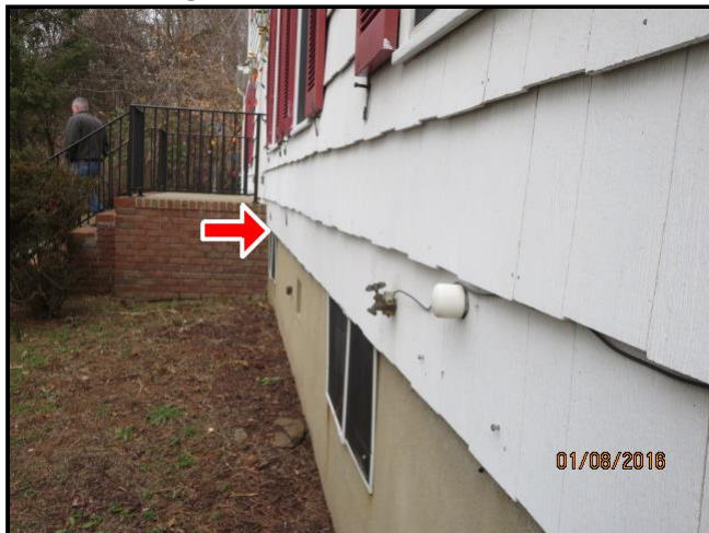
2.0 Item 9(Picture) Buckled siding
