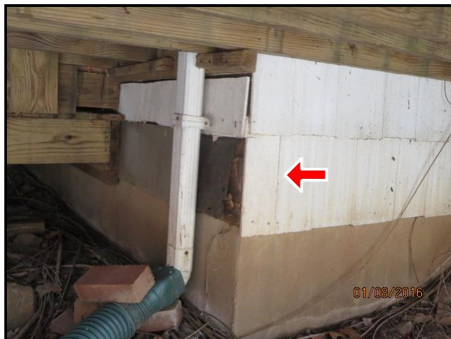
2.0 Item 10(Picture) Wood rot
