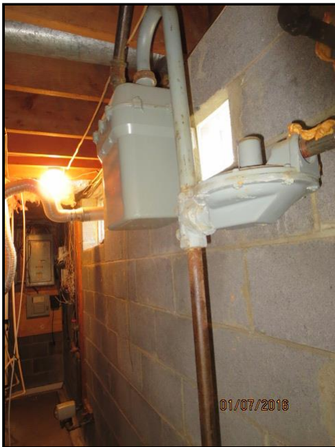
5.5 Item 1(Picture) Gas meter
