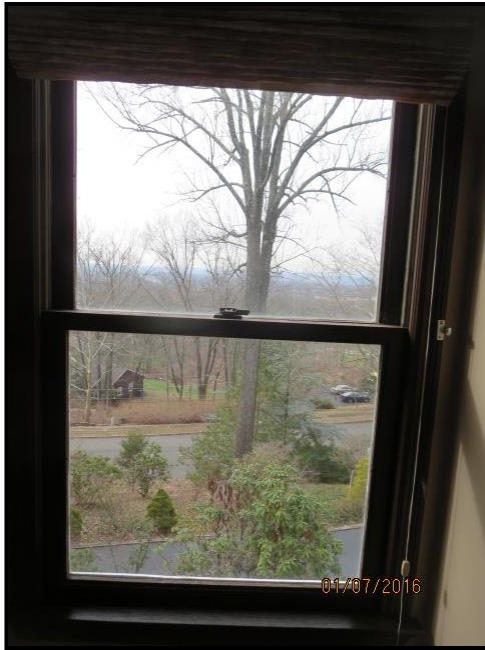
8.6 Item 2(Picture) Non working window
