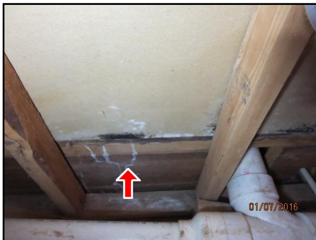
6.0 Item 2(Picture) Possible mold
