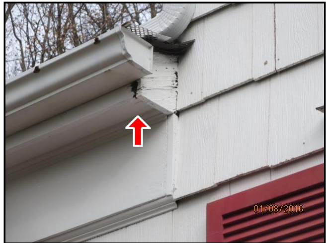
2.0 Item 8(Picture) Rotted trim
