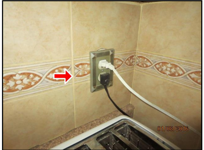
3.3 Item 11(Picture) Non GFCI
