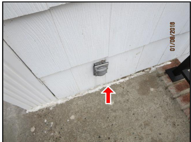
3.3 Item 6(Picture) open ground and loose
