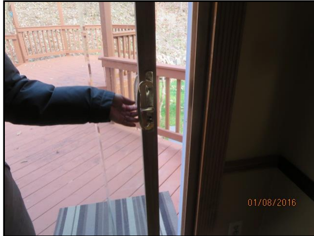
8.5 Item 2(Picture) Broken lock
