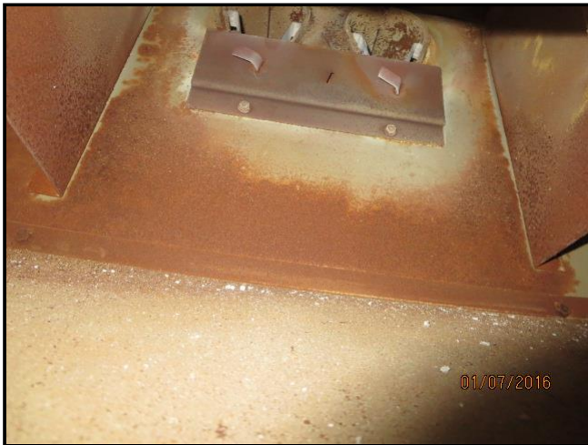
4.0 Item 3(Picture) Rust
