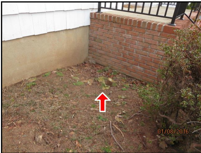
2.4 Item 1(Picture) Negative slope
