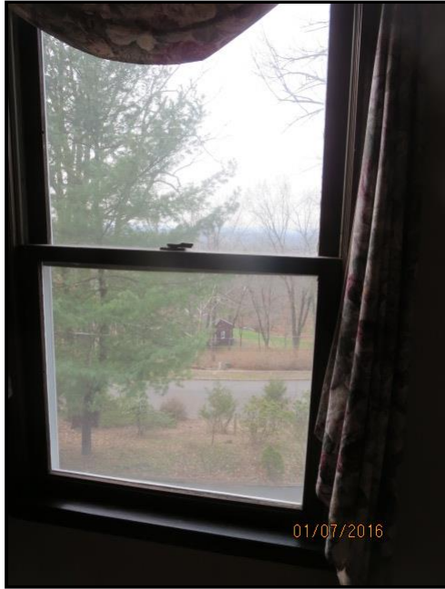
8.6 Item 1(Picture) Non working window
