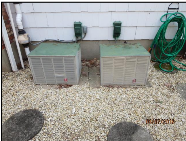
4.8 Item 1(Picture) Condensers
