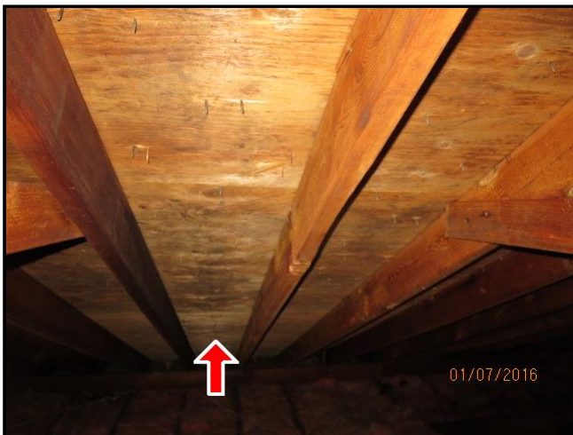
6.5 Item 3(Picture) Possible Mold
