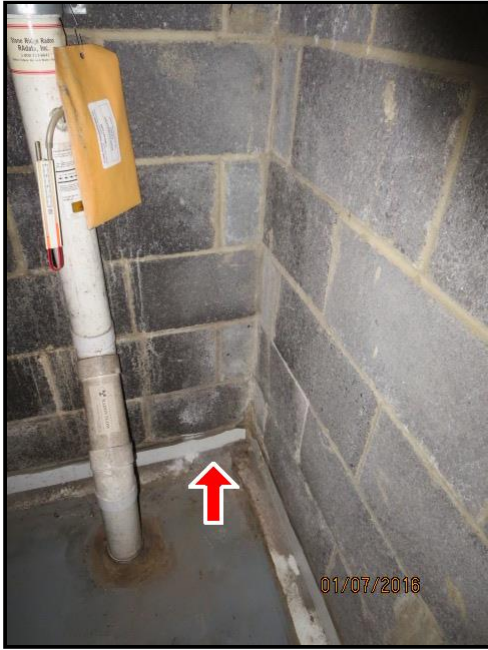
6.0 Item 3(Picture) Efflorescence
