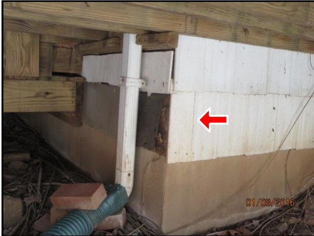
2.0 Item 10(Picture) Wood rot
