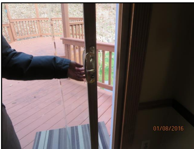
8.5 Item 2(Picture) Broken lock
