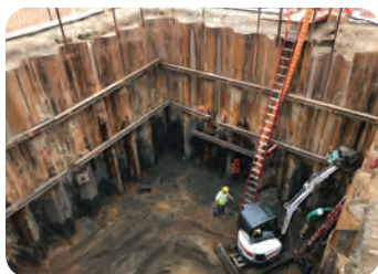
Edison Pump Station, NJ
