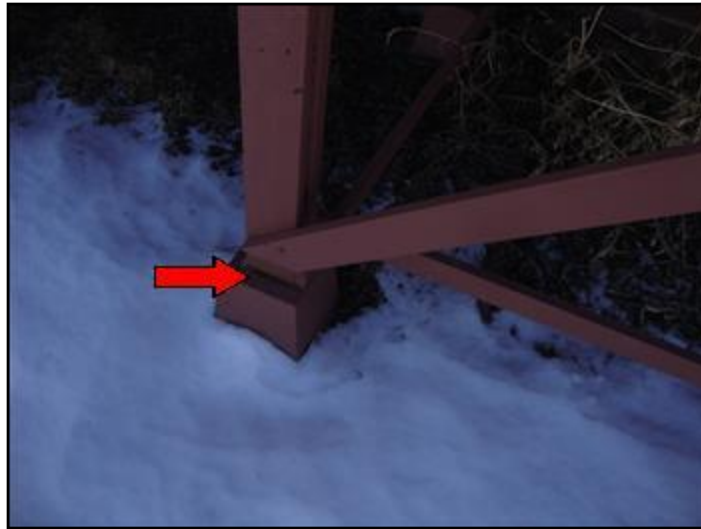
82. Loose support at the base
