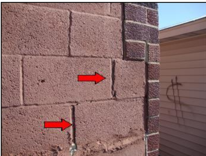
50. Settlement cracks noted
