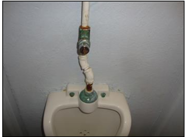
16. Evidence of past leakage noted
