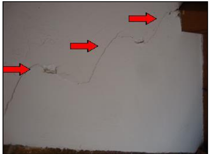
47. Settlement cracks noted
