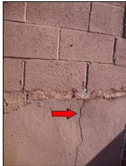
49. Settlement cracks noted
