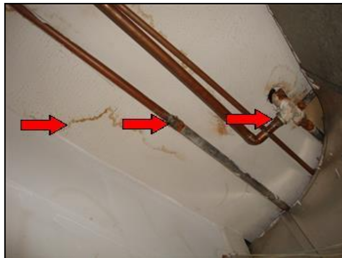
17. Evidence of past leakage noted
