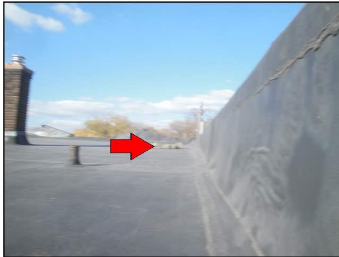
6. Debris/oil on roof
