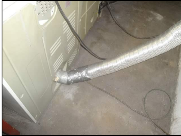
140. Dryer vent material not smooth wall
