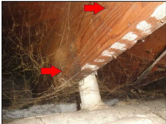
65. Split or damaged
