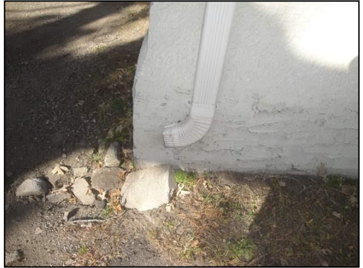
23. Downspouts end too close to building
