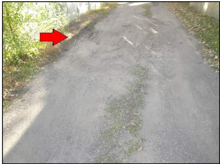
47. Improper slope or drainage
