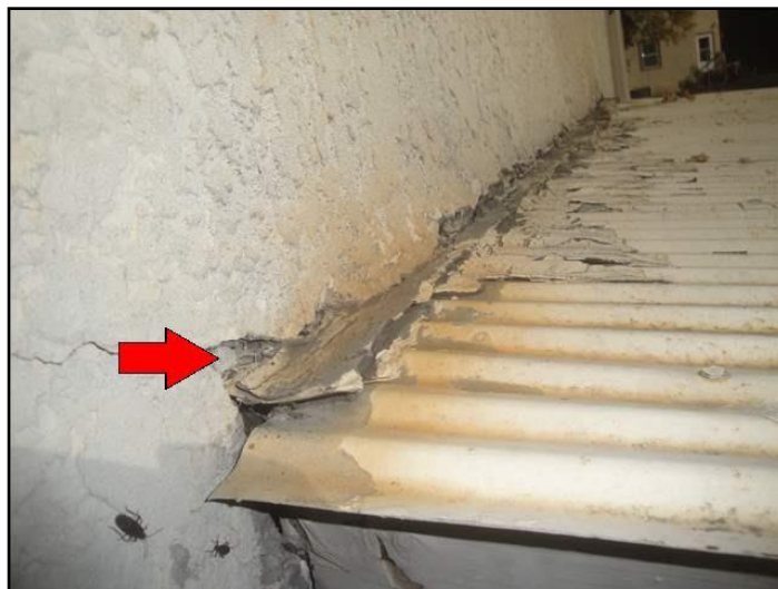
2. Loose, damaged, patched, open seams
