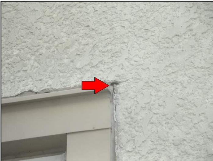
28. Caulking missing or ineffective
