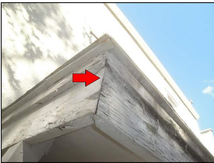
25. Paint or stain needed
