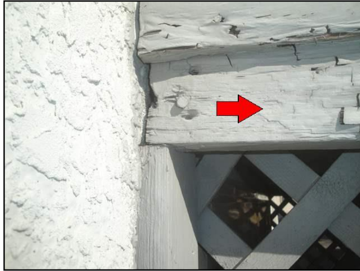
27. Paint or stain needed
