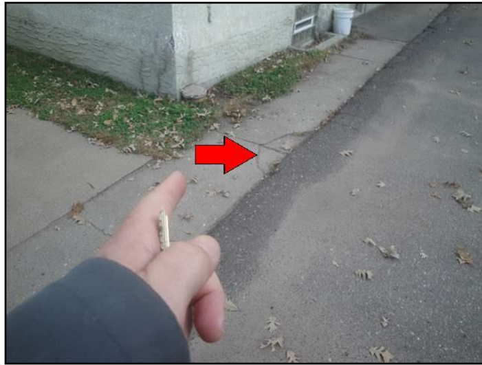
48. Cracked or damaged surfaces
