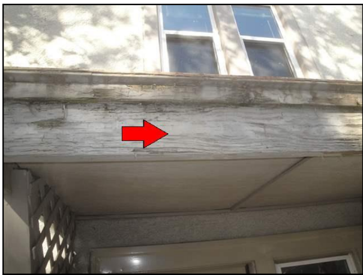
26. Paint or stain needed
