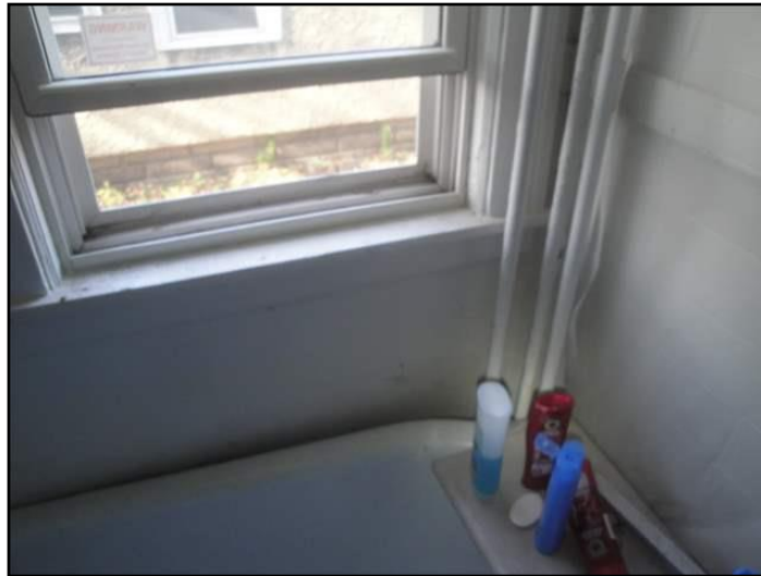
118. Safety glass not installed
