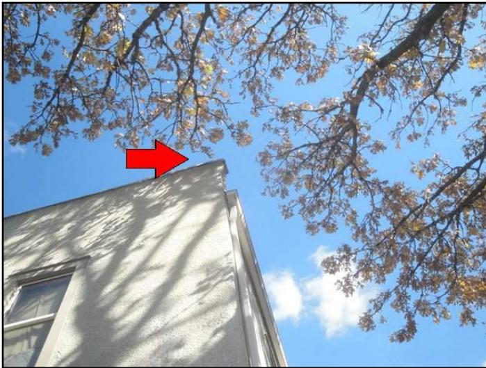
53. Trees or shrubs too close to building
