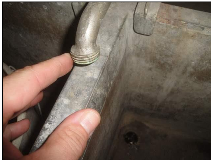
97. Air gap defective
