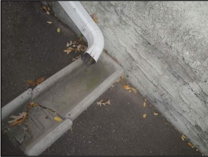
22. Downspouts end too close to building
