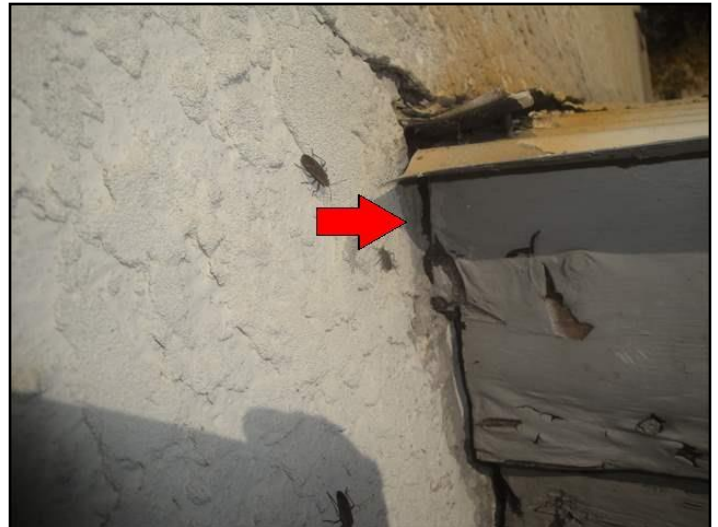
29. Caulking missing or ineffective
