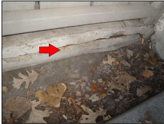
63. Spalling, crumbling or broken material
