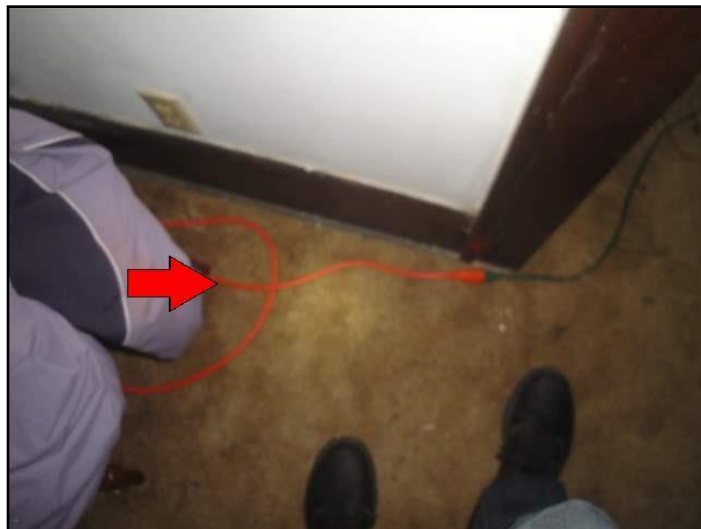
68. Extension cord used as permanent wiring
