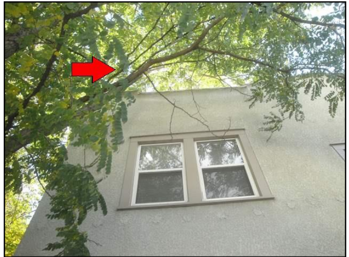
54. Trees or shrubs too close to building
