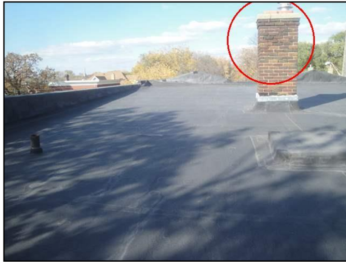
81. Loose, missing or deteriorated mortar
