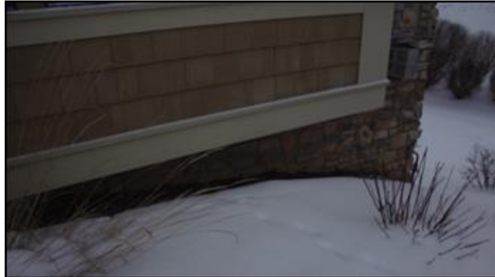
Too close to grade
