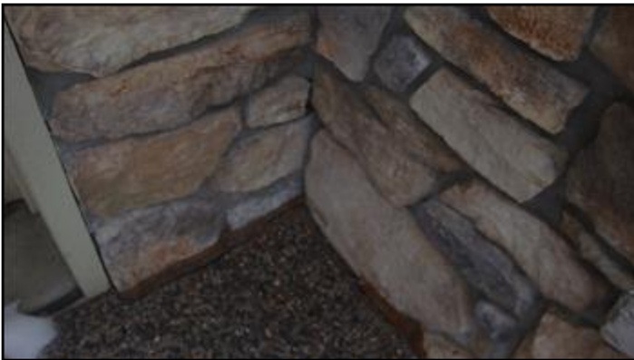
Missing, ineffective weep holes or flashings
