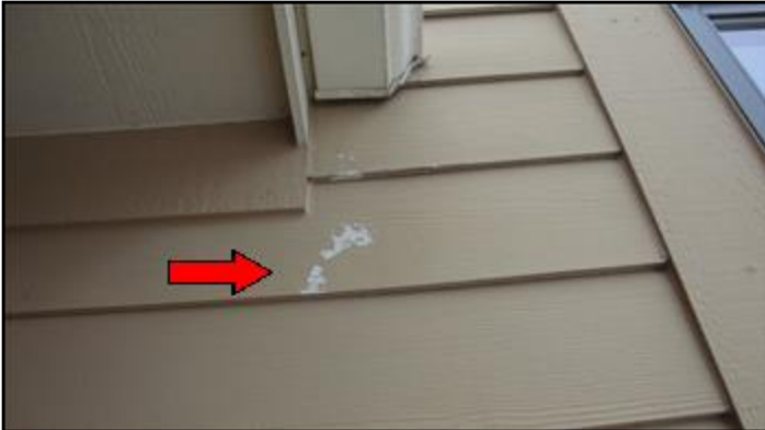
Too close to grade
