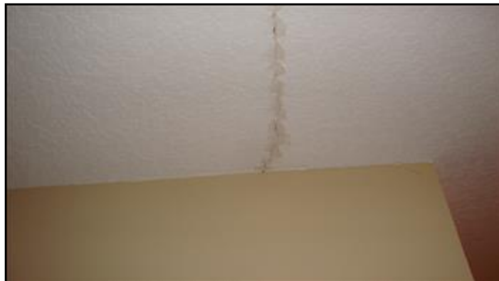
Typical minor settlement
