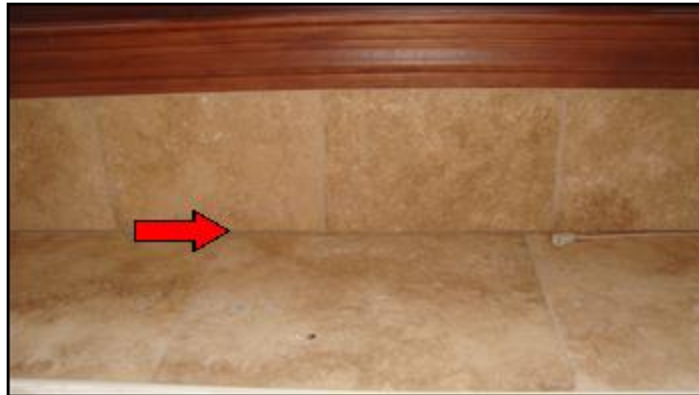
Grout loose, missing or deteriorated
