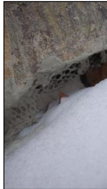
Missing, ineffective weep holes or flashings
