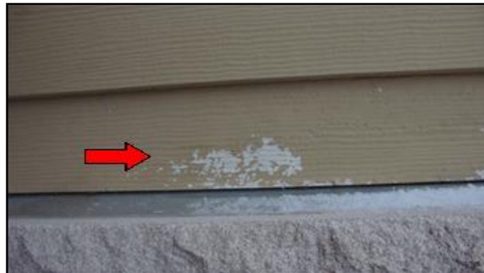
Missing paint or caulking
