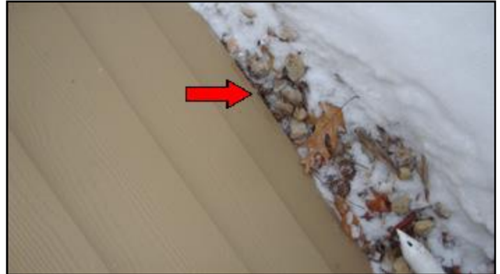
Too close to grade
