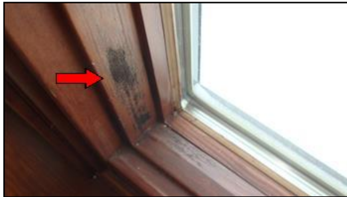
Paint or stain needed
