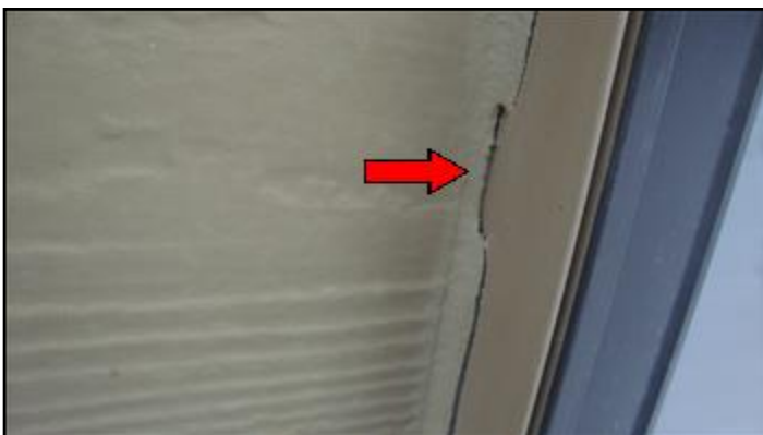
Caulking missing or deteriorated
