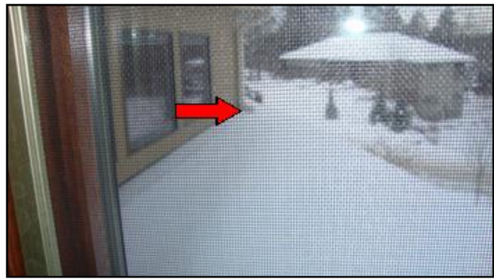
Downspouts discharging onto roofs
