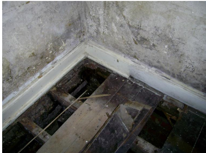
2 Bouncy floor boards indicated a defect - the embedded timber joists had suffered from wet rot and death watch beetle attack
